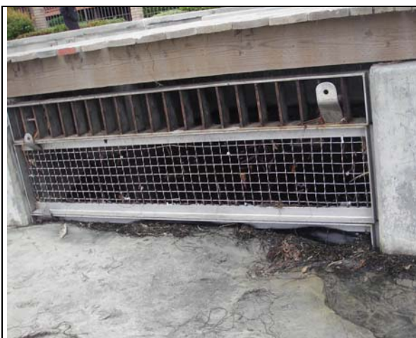
Figure 12. A storm water catchment basin located on the beach at Avenida de la Playa.
