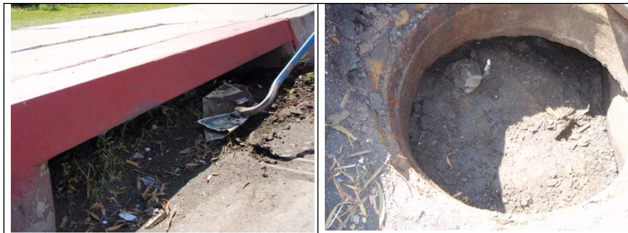
Figure 3-12. Storm Drain Inlet with Dirt and Debris (southwest corner of 32 nd Street and Commercial Street)
