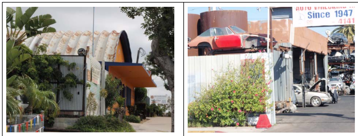
Figure 3-9. Facilities with Metal Structures in Poor Condition (rust and staining evident)
