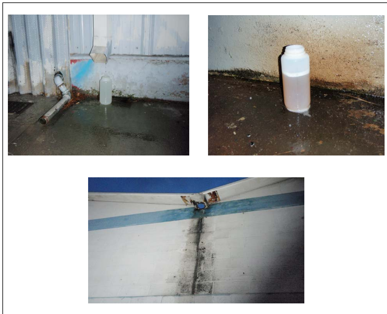
Figure 2-4. Rooftop Runoff Samples from Locations with Observed Surface Stains
