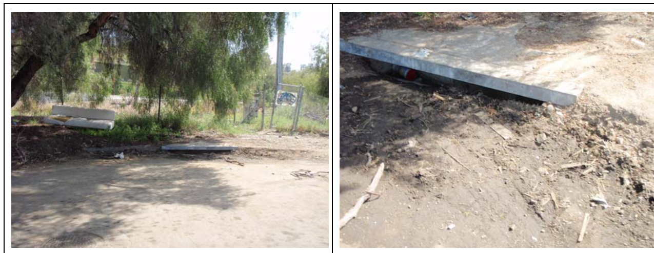
Figure 3-13. Storm Drain Inlet with Dirt and Debris Drains Directly into Chollas Creek (38 th Street and Ash Street)
