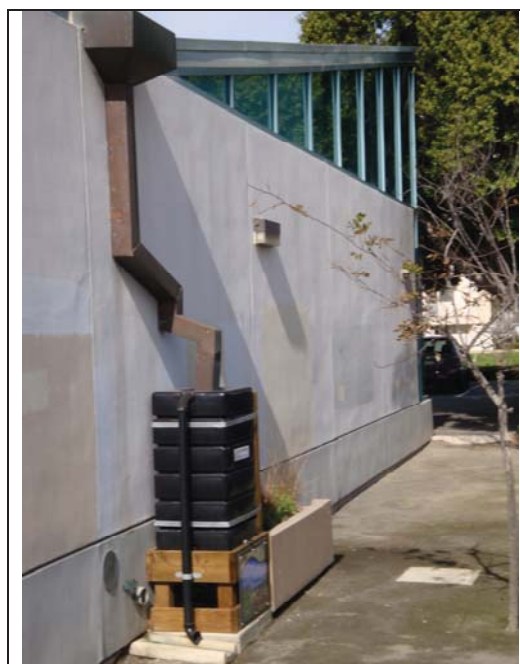
Figure 4. Brown Copper Downspout at Mira Mesa Library with Rain Barrel Downspout Disconnect System and Adjacent Infiltration Area
