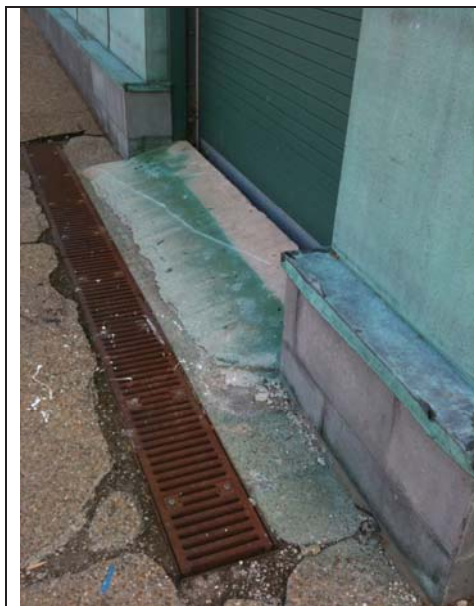
Figure 1. Copper salt staining from a copper-clad building, Brandeis University, Boston, Massachusetts (Quigley, 2011)
