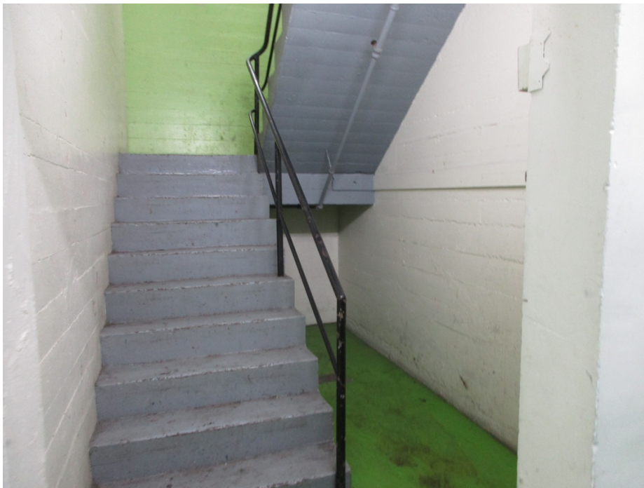
Figure 20: Interior view showing an original concrete stair with steel pipe railings. The stairs will be removed.
