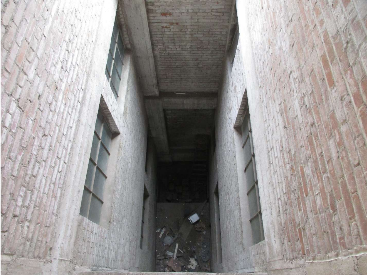
20 THE INTERIOR OF THE LIGHTWELL AT THE WEST SIDE OF THE EAST WING, LOOKING DOWN.
