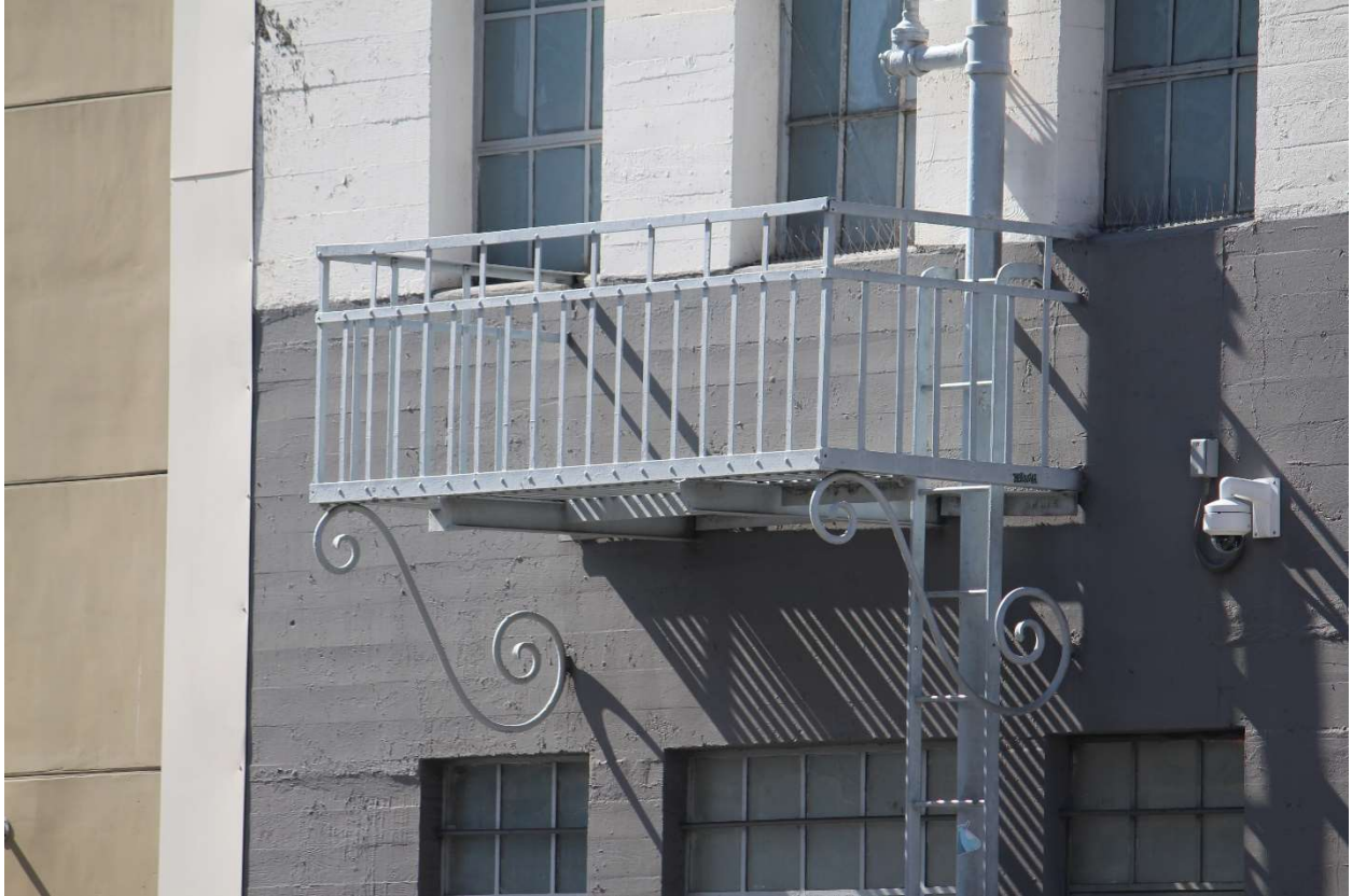
11 ORIGINAL STEEL FIRE-ESCAPE BALCONY AT THE SOUTHERN END OF THE EAST FACADE.
