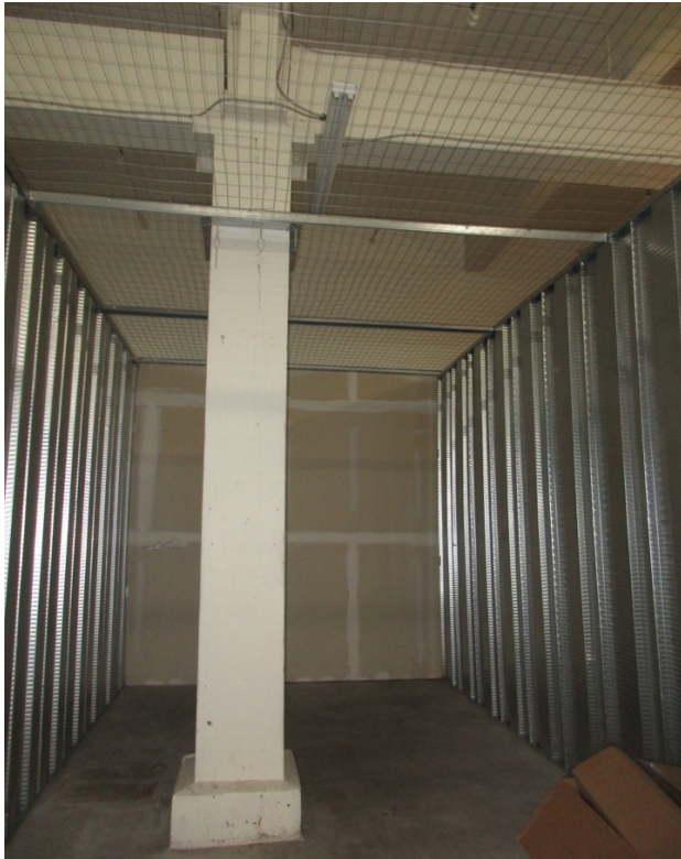
Figure 19: Interior view showing a typical storage space and original post and beam construction. These will be removed.
