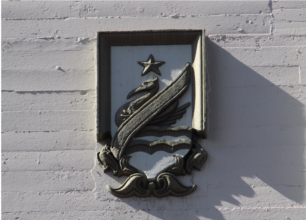
Figure 15: One of three cast-stone “pelican shields” that will be protected-in-place. Note the adjacent board-formed cast-in-place concrete wall finish.
