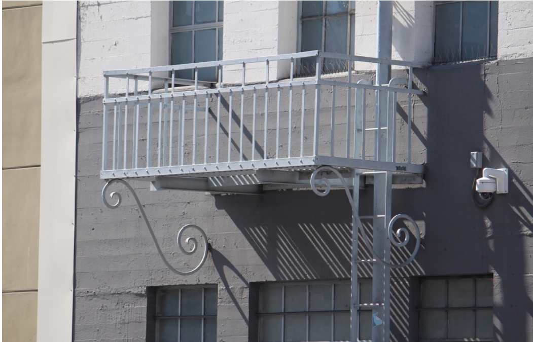
Figure 17: One of two fire escape balconies on the east facade with scrolled bracket supports. These will be incorporated into the rehabilitated facade.
