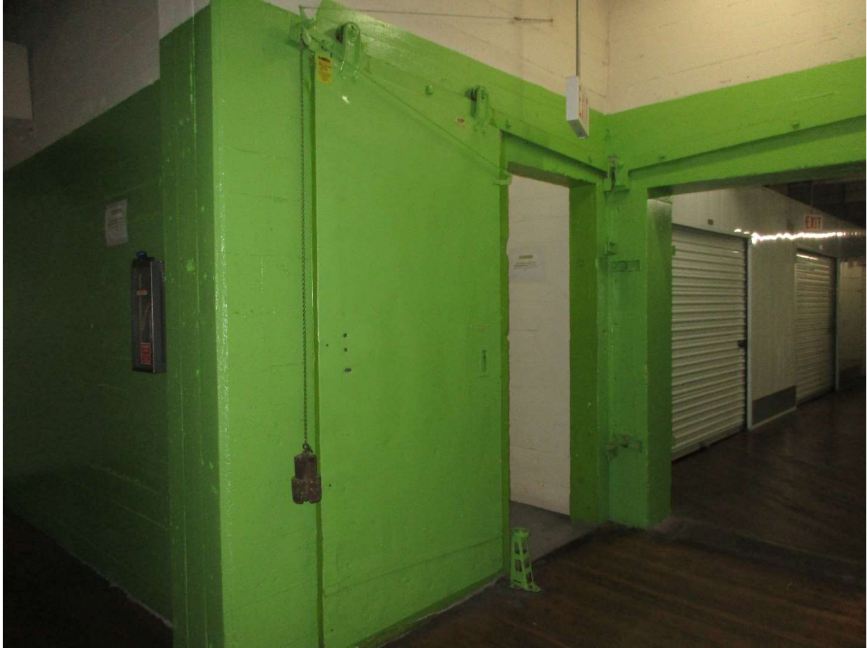
19 LOOKING NORTH AT THE BARN-TYPE FIRE DOOR FOR THE CENTRAL STAIR CORE ENTRY AT THE THIRD FLOOR. THE CHAIN WEIGHT AND PULLEY SYSTEM ARE ALSO VISIBLE.
