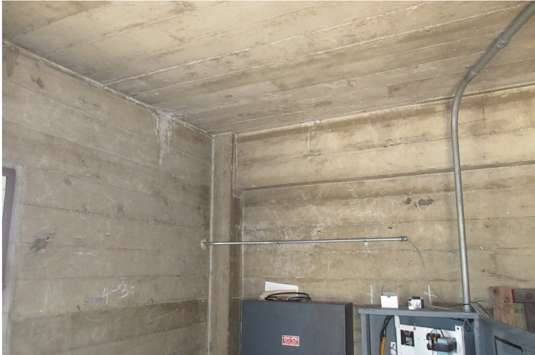
Figure 7: View of the interior of an elevator equipment room on the roof where the original yellow/beige integral concrete color is exposed. Aside from soiling, this is the original color of the building's exterior walls.
