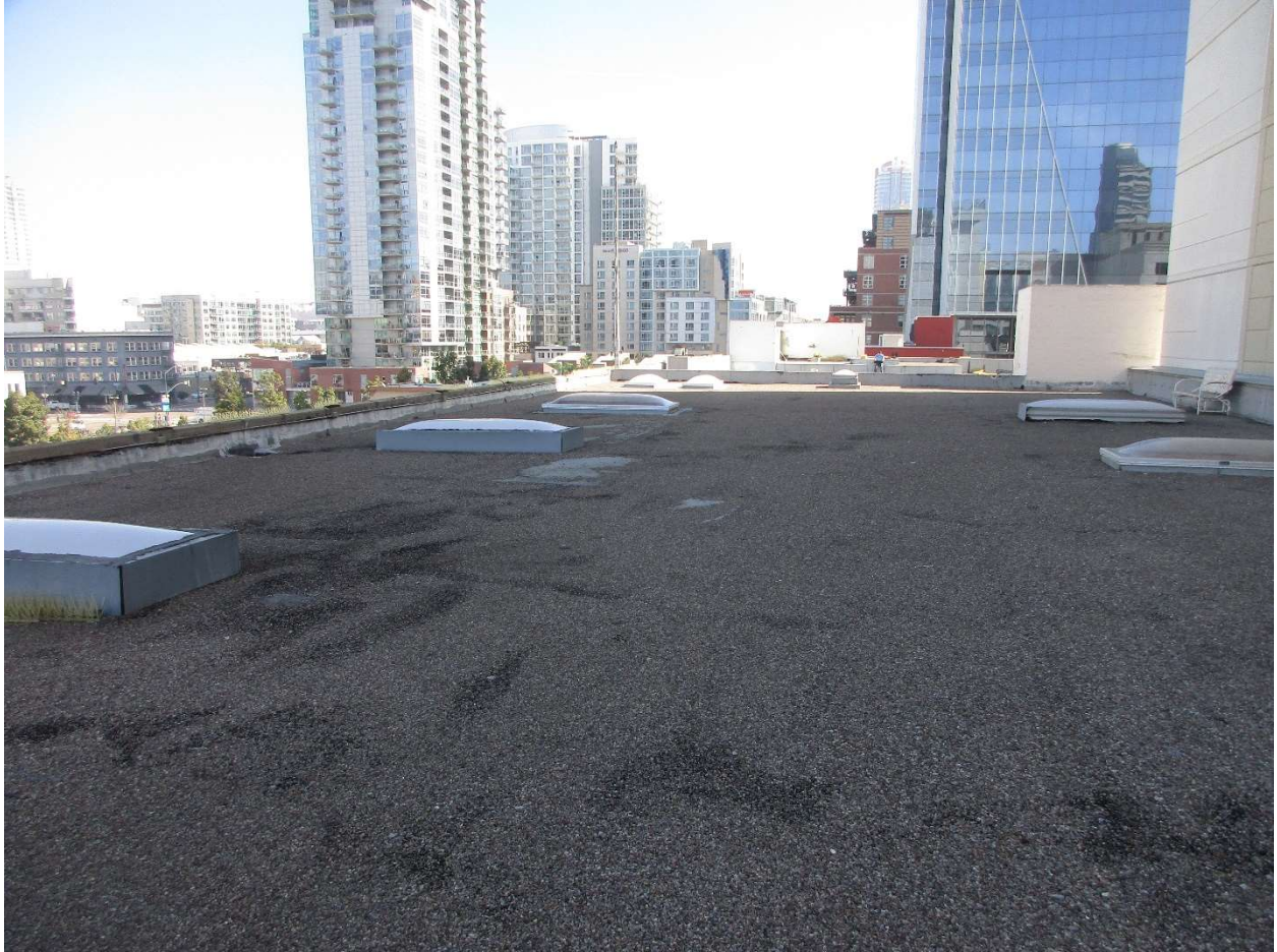
21 VIEW LOOKNG EAST OVER THE ROOF FROM THE WEST END OF THE WEST WING.
