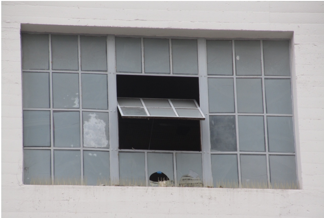
Figure 10: Typical historic steel window with putty-set glazing. Note the added film on the glass. Replace broken and missing glass and restore windows to working condition.
