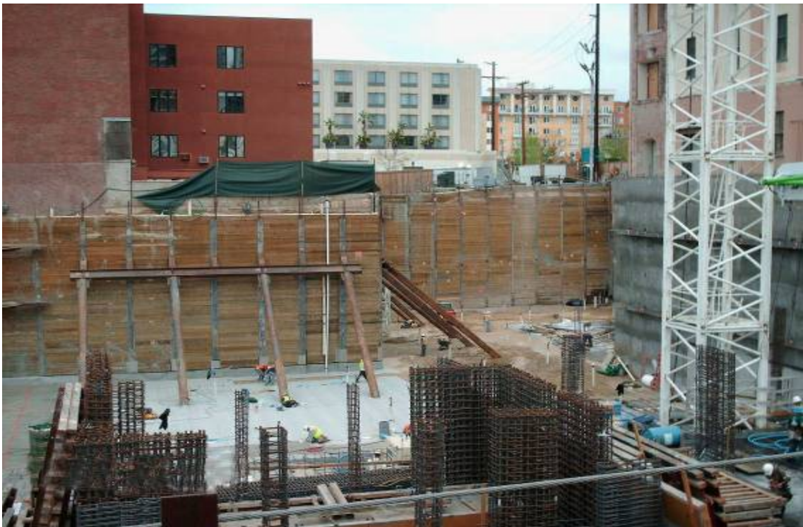
Temporary shoring consisting of internal bracing, tie-back anchors, and soil nail anchors, Downtown San Diego
