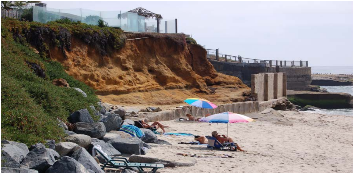
Coastal erosion protection in Ocean Beach. Note recession between seawall and bluff face.
