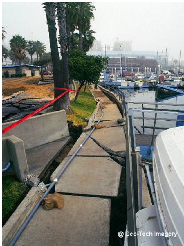
Liquefaction and lateral spread at Redondo Beach Marina parking lot, Northridge Earthquake 1994
