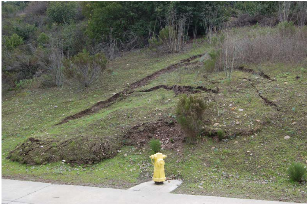
Surficial slope failure after heavy rainfall December 2010
