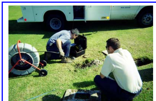
A typical CCTV investigation of a sewer lateral line in Mission Bay Park
