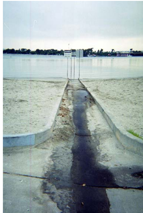
Un-diverted storm drain at Bahia Point
