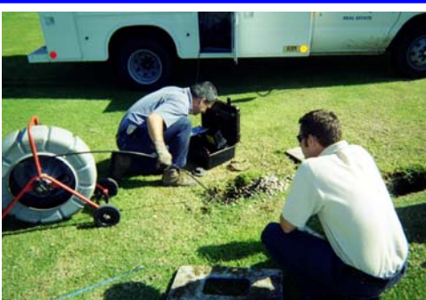
A typical CCTV investigation of a sewer lateral line in Mission Bay Park
