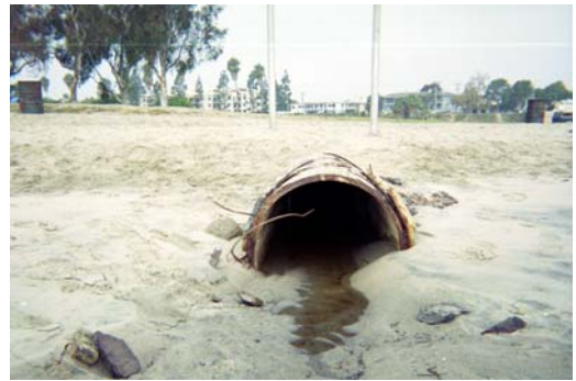
Storm Drain SD5-2 conveys irrigation runoff to Wildlife Refuge
