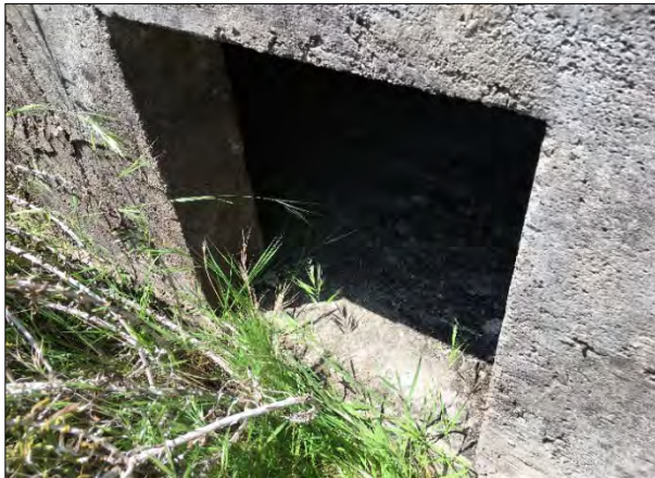
A side access portal on lower flue
