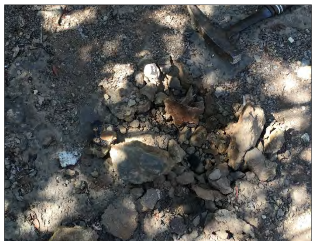
Friable concrete foundation - ore roaster area.
