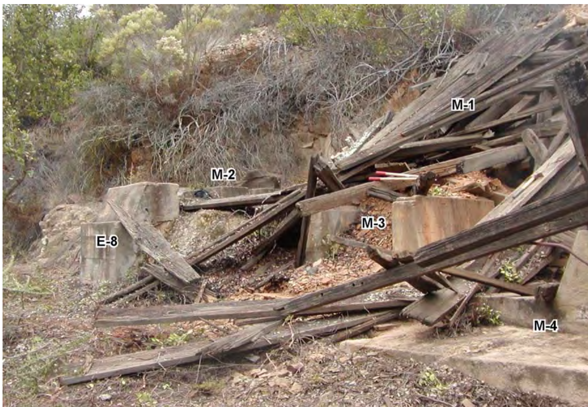
Figure 6. Core processing area showing the collapsed ore bin (M-1), and concrete footings for machinery used in ore processing.
