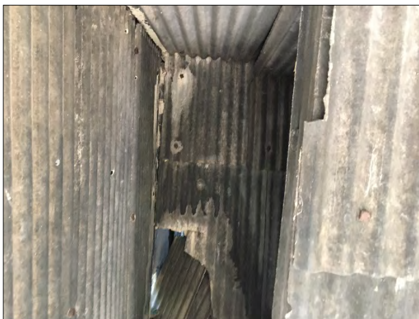
Interior asbestos baffles in dust flue.
