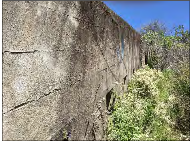
Northern side of flue showing access portals. Side access portal on flue
