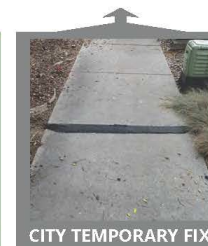
CITY TEMPORARY FIX
