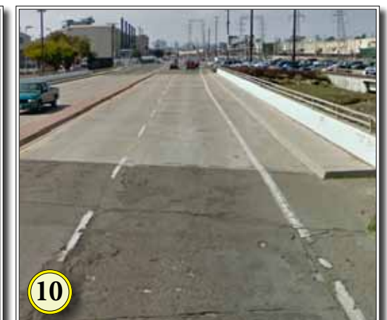
10 Concrete and asphalt conditions are poorest in the middle and southern segment of the corridor
