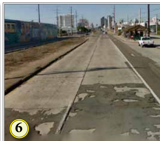
6 Areas where asphalt has been used over the concrete surface, are in very poor condition
