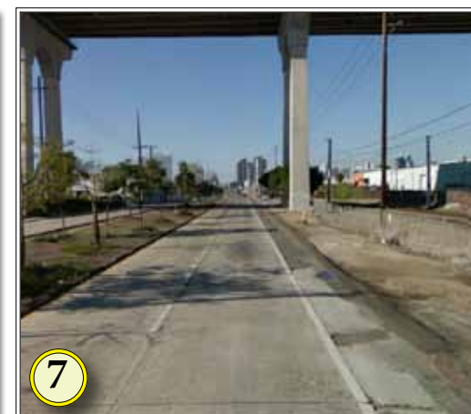
7 The shoulders where most cyclist have to ride, are in very poor condition with safety issues
