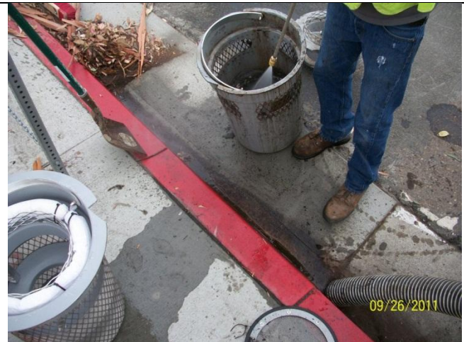
D. Remove DII basket from catch basin and pressure wash in gutter, vacuum wash water
