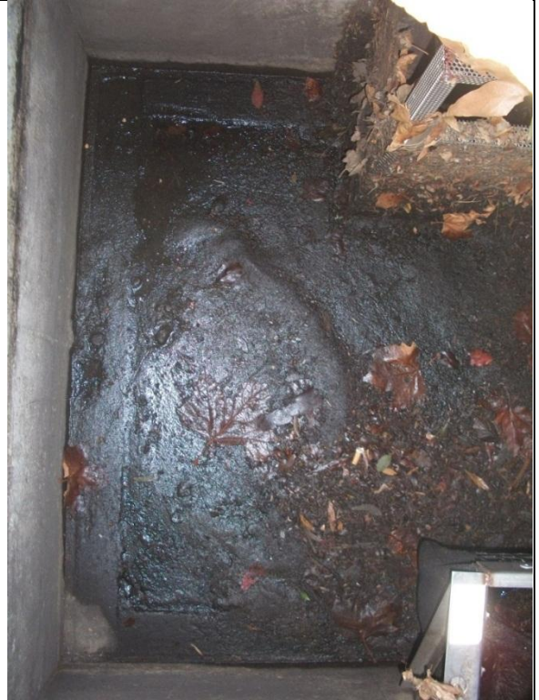
D. Catch basin floor from above
