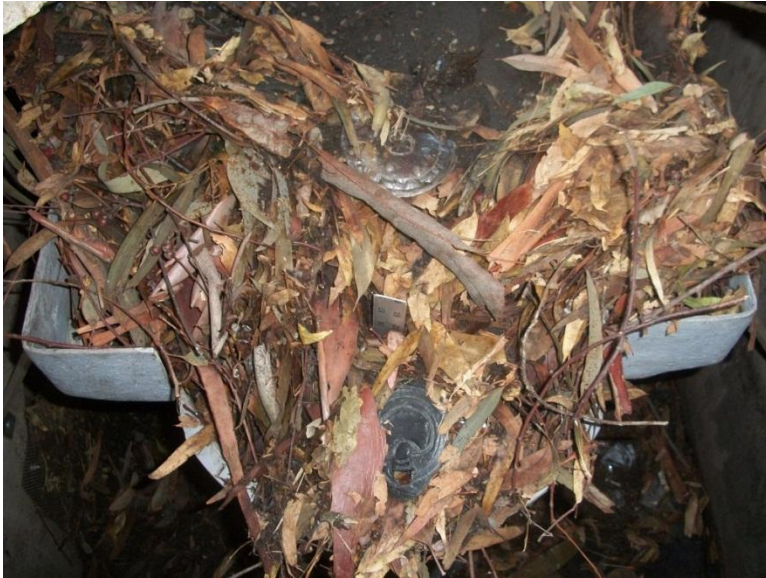
A. Curb inlet basket and collection tray from above
