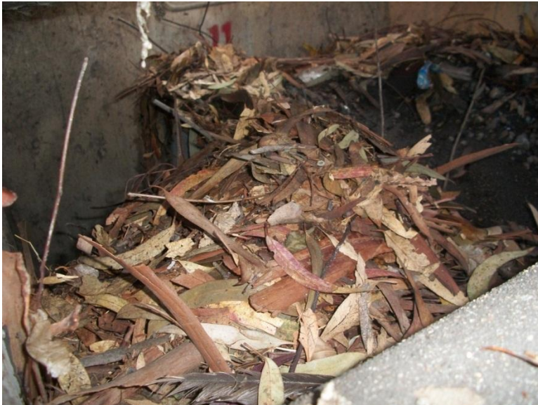
C. Curb inlet basket and collection tray from street
