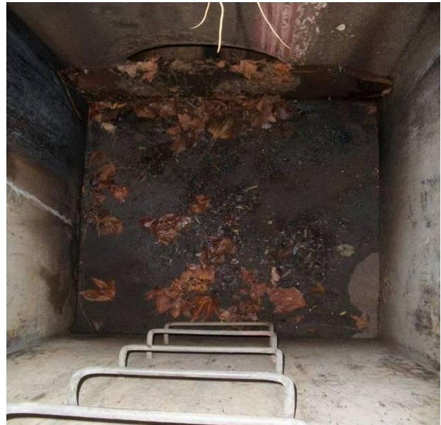
d) Post-storm inspection- Presence of gross solids in catch basin and on top of outlet screen.
