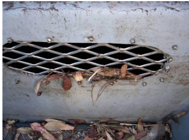
d) Post-storm inspection- Accumulation of gross solids on bypass orifice of filter basket.
