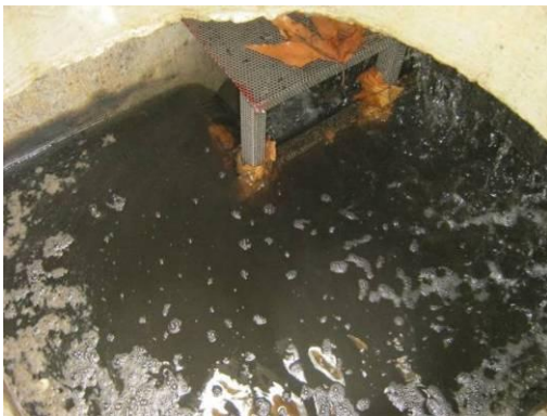
c) Bypass of CPS; gross solids exiting through overflow.
