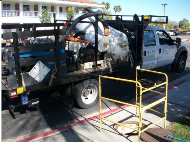
A. Park vac truck, close lane, open manhole and stage pedestrian barricade
