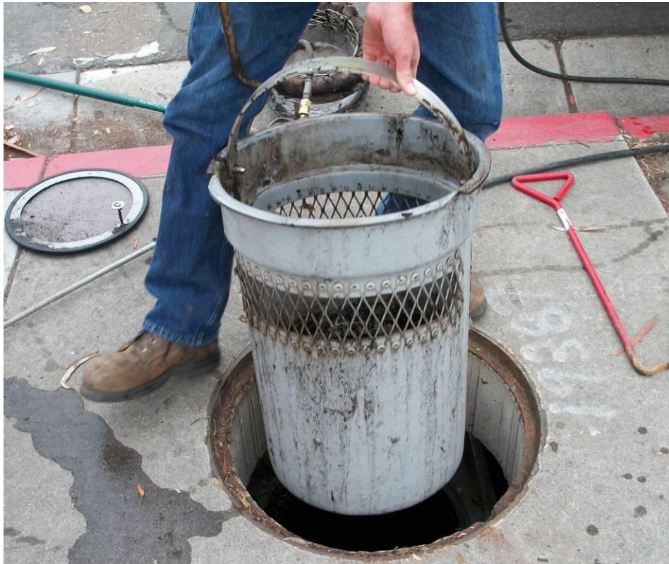
Figure 2-4. Bio Clean Round Curb Inlet Basket Removed from Manhole
