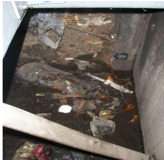
d) Post-storm inspection- Bypass of gross solids evident; Presence of gross solids in catch basin and on outlet screen.
