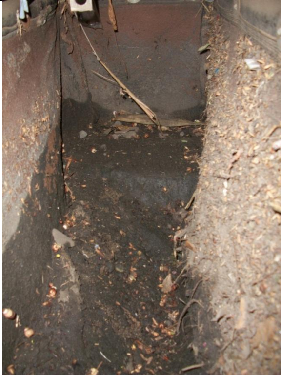
A. Curb inlet basket from side
