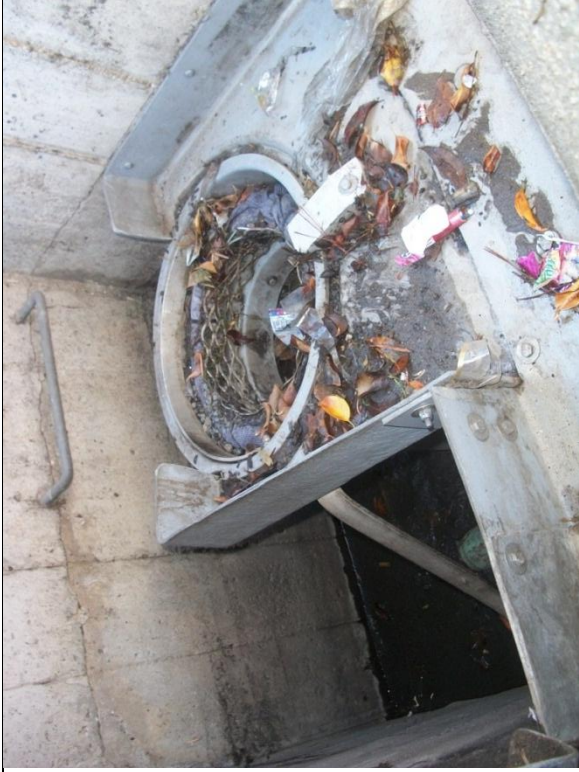
A. Curb inlet basket and collection tray from street
