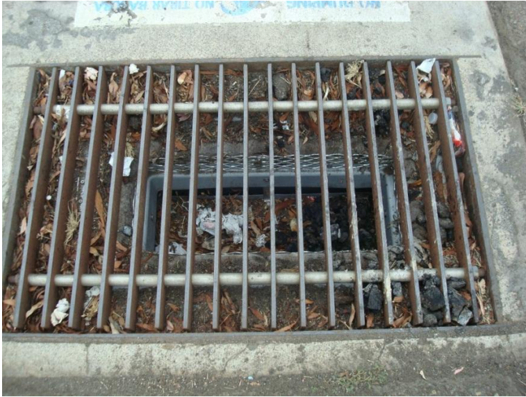
A. Grate inlet basket and skimmer insert from above, full
