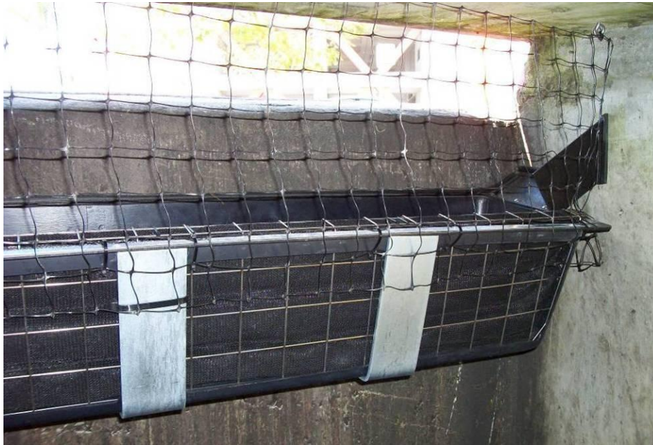
Figure 2-19. REM Triton Curb Inlet Filter Insert Installed at PET Site
