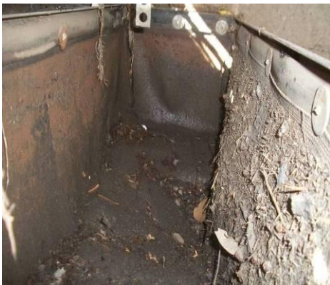
e) Post-storm inspection- Sediment and organic debris clogging basket fabric.
