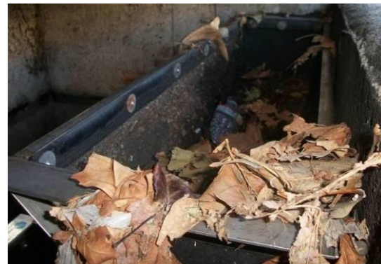
d) Post-storm inspection- Evidence of gross solids overtopping basket; sediment and organic debris clogging fabric.
