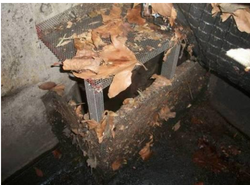
e) Post-storm inspection- Evidence of gross solids bypass of CPS; clogging of CPS with sediment and organic debris.
