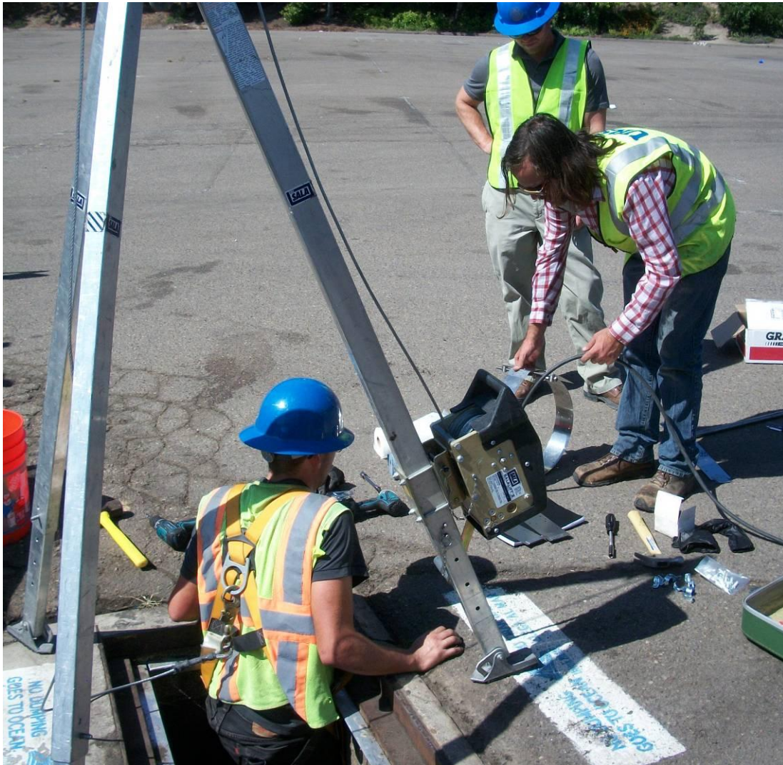
Figure 3-5. Installation of Flow Meter at Bio Clean QUAL Pilot Site
