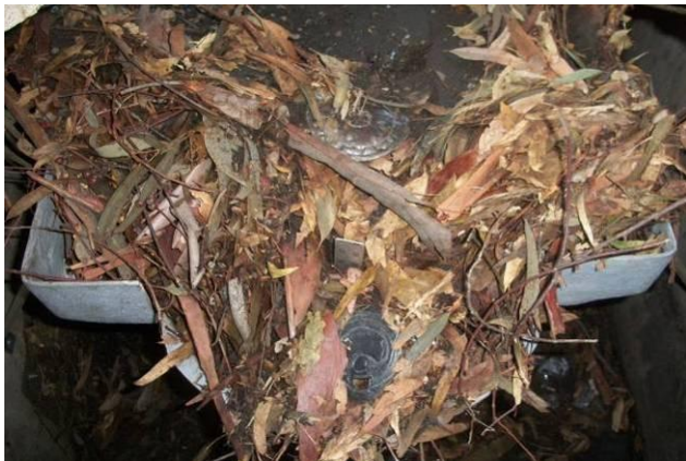
c) Post-storm inspection- Over 100% full of gross solids, largely organic debris and sediment.
