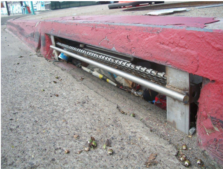
C. ARS from street, debris trapped beneath screen
