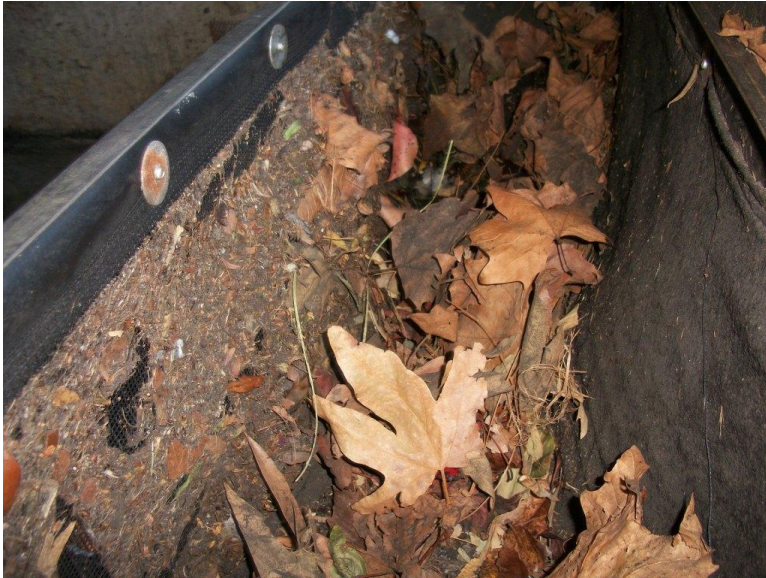
A. Curb inlet basket from side
