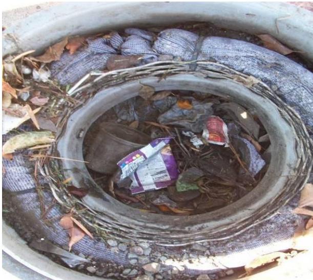
c) Post-storm inspection- Product nearly full of gross solids.
