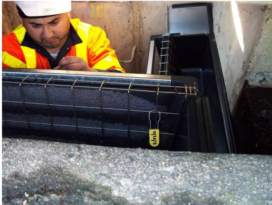
Figure 2-17. Configuration of the REM Triton Curb Inlet Filter Inserts at BER-PL Site
