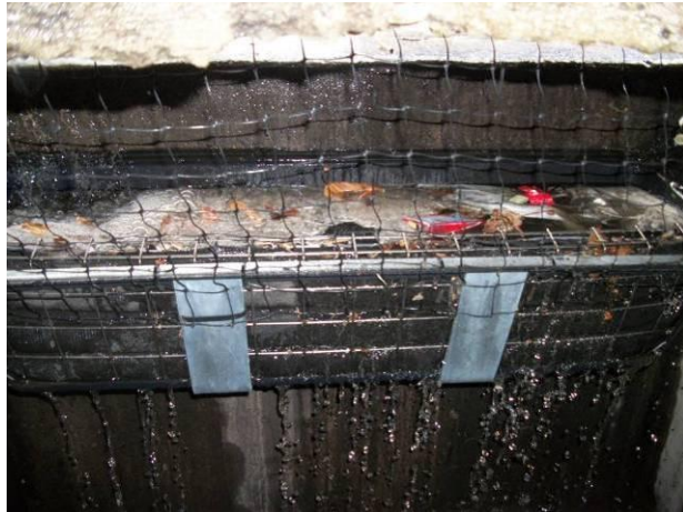
a) Before initial bypass; product full of water.
