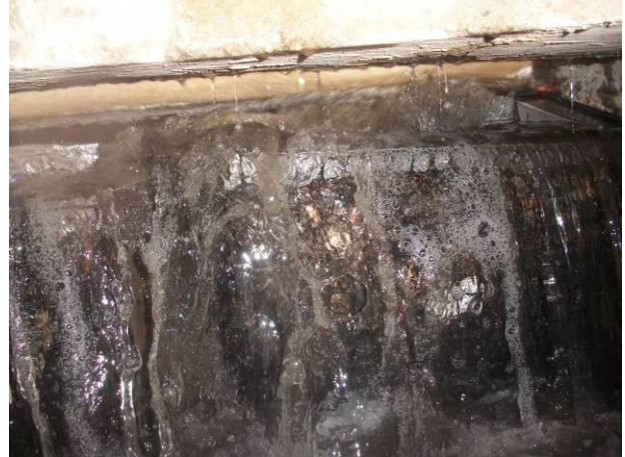
b) Flow bypass of BMP- Right basket
