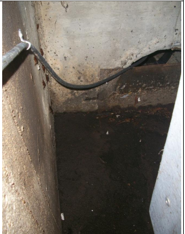
D. Catch basin floor from above, roaches at left
