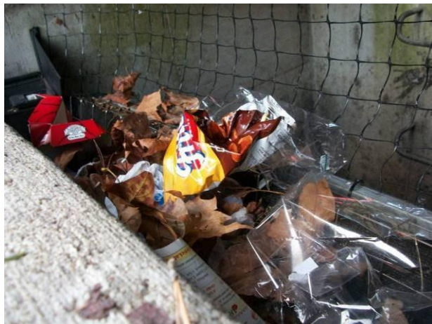
c) Post-storm inspection- Product nearly full of gross solids; larger gross solids retained by webbing.
