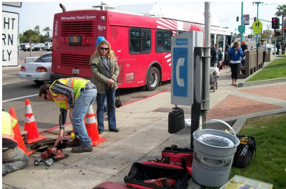
Figure 2-6. Installation of Bio Clean Round Curb Inlet Basket at ECB-54 Pilot Site
