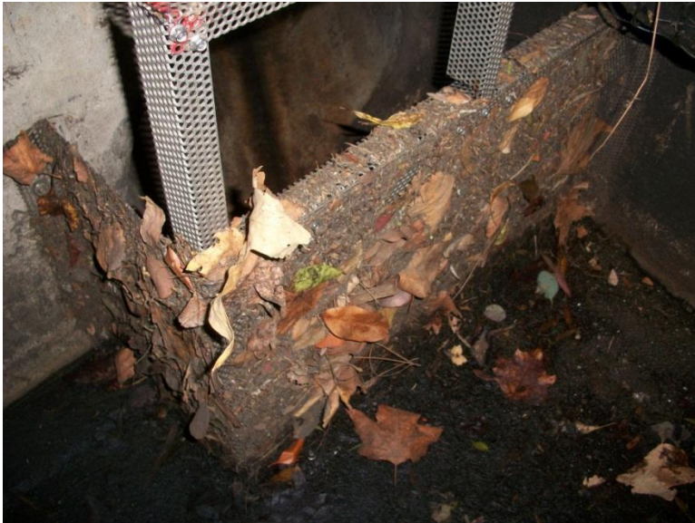
C. CPS from inside catch basin
