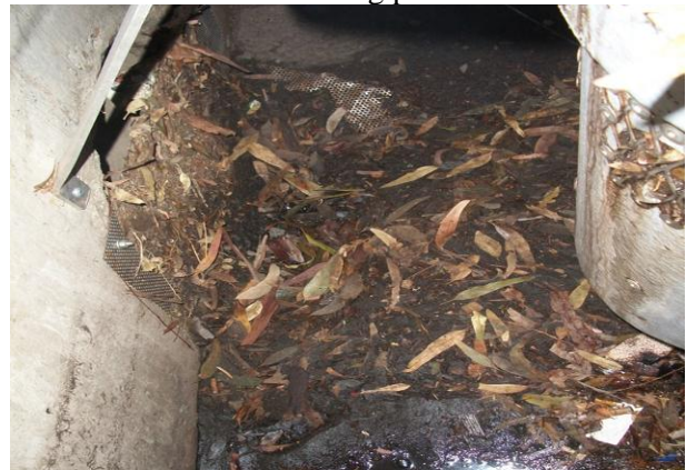
d) Post storm inspection- Presence of gross solids in catch basin. Note gross solids on top of outlet pipe screen.
