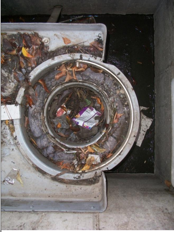
B. Curb inlet basket and media boom from above
