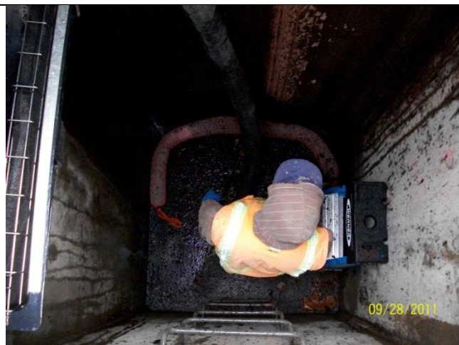
E. Vacuum DII wash water from catch basin floor
