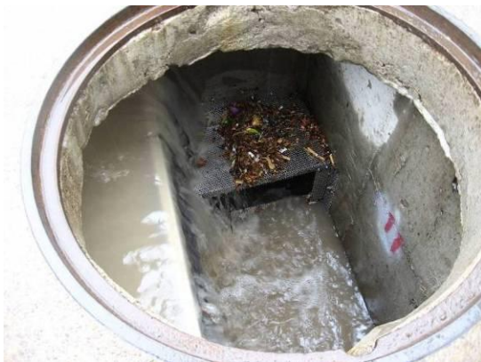
c) Flow bypass of basket (on left) and CPS.
