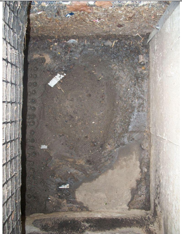
D. Catch basin floor from above
