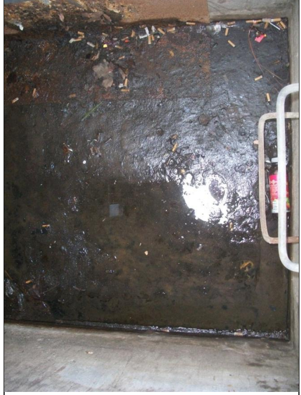
D. Catch basin floor from above
