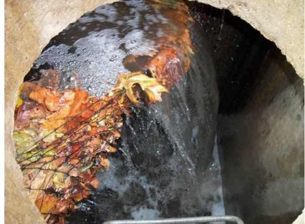
b) Flow bypass of BMP; top of webbing unsecured allowing bypass of gross solids.
