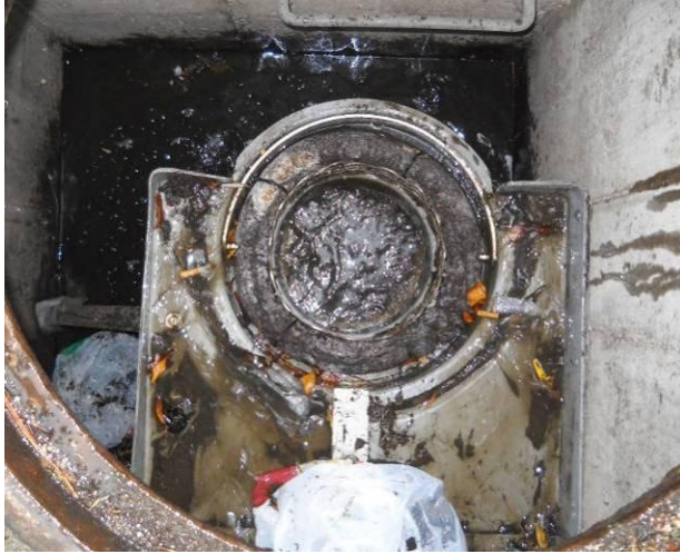
a) Before initial bypass- Product full of water.
