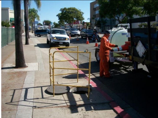
A. Park vac truck, close lane, open manhole and stage pedestrian barricade
