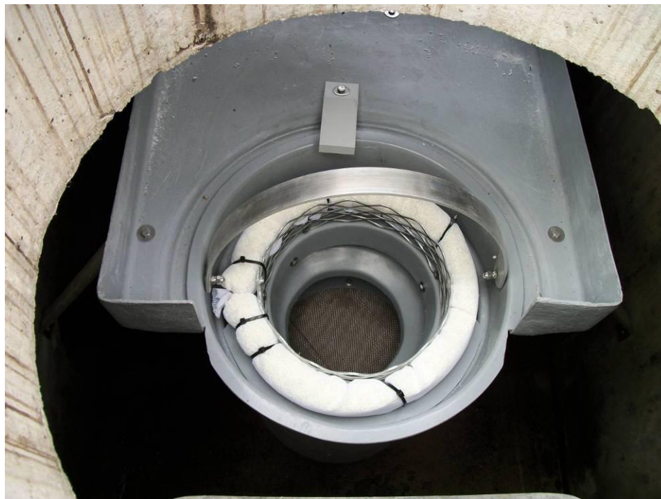
Figure 2-3. Bio Clean Round Curb Inlet Basket and Shelf System Installed at BEY-TS.
