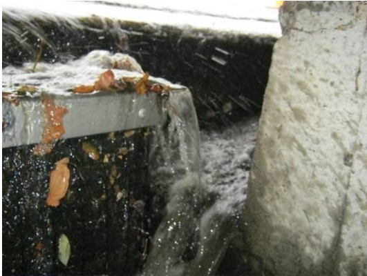
a) Initial bypass of BMP- Curb inlet basket shown from inside catch basin.
