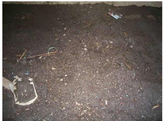
d) Post-storm inspection- Large amount of sediment present in catch basin.
