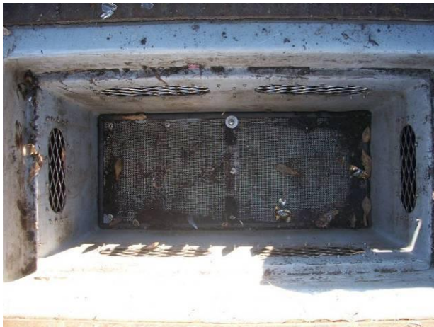
c) Post-storm inspection- Screen on bottom of filter basket; minimal gross solids present.
