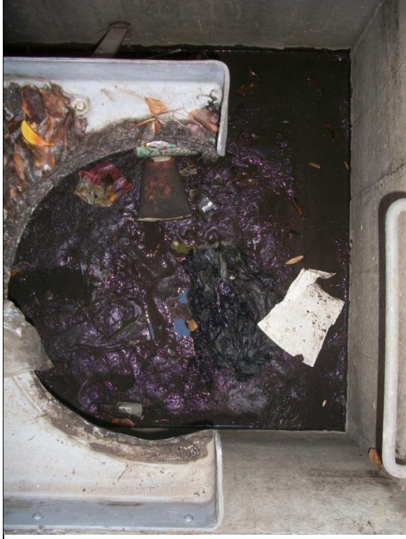
D. Catch basin floor from above
