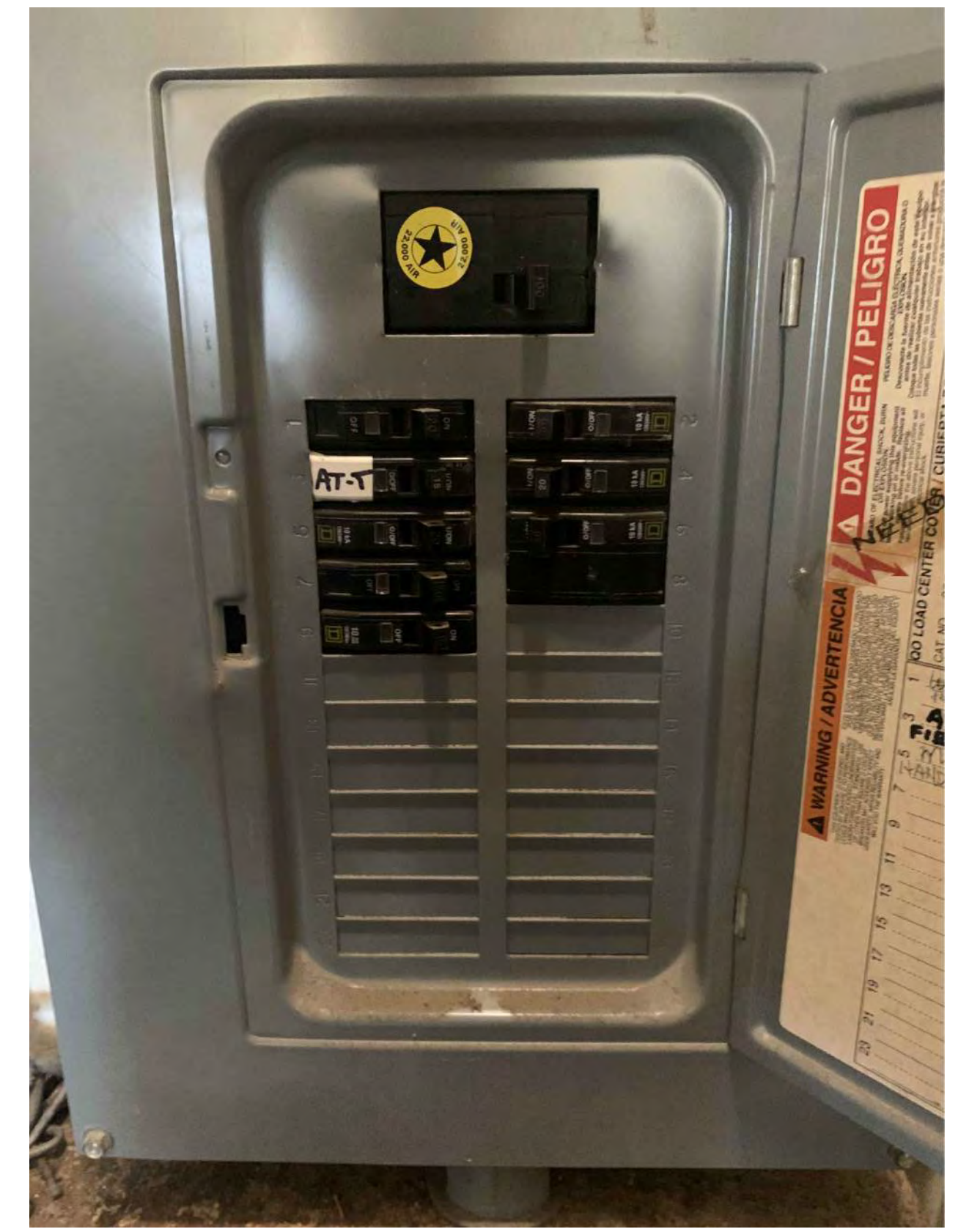
EXISTING PANEL HP2
