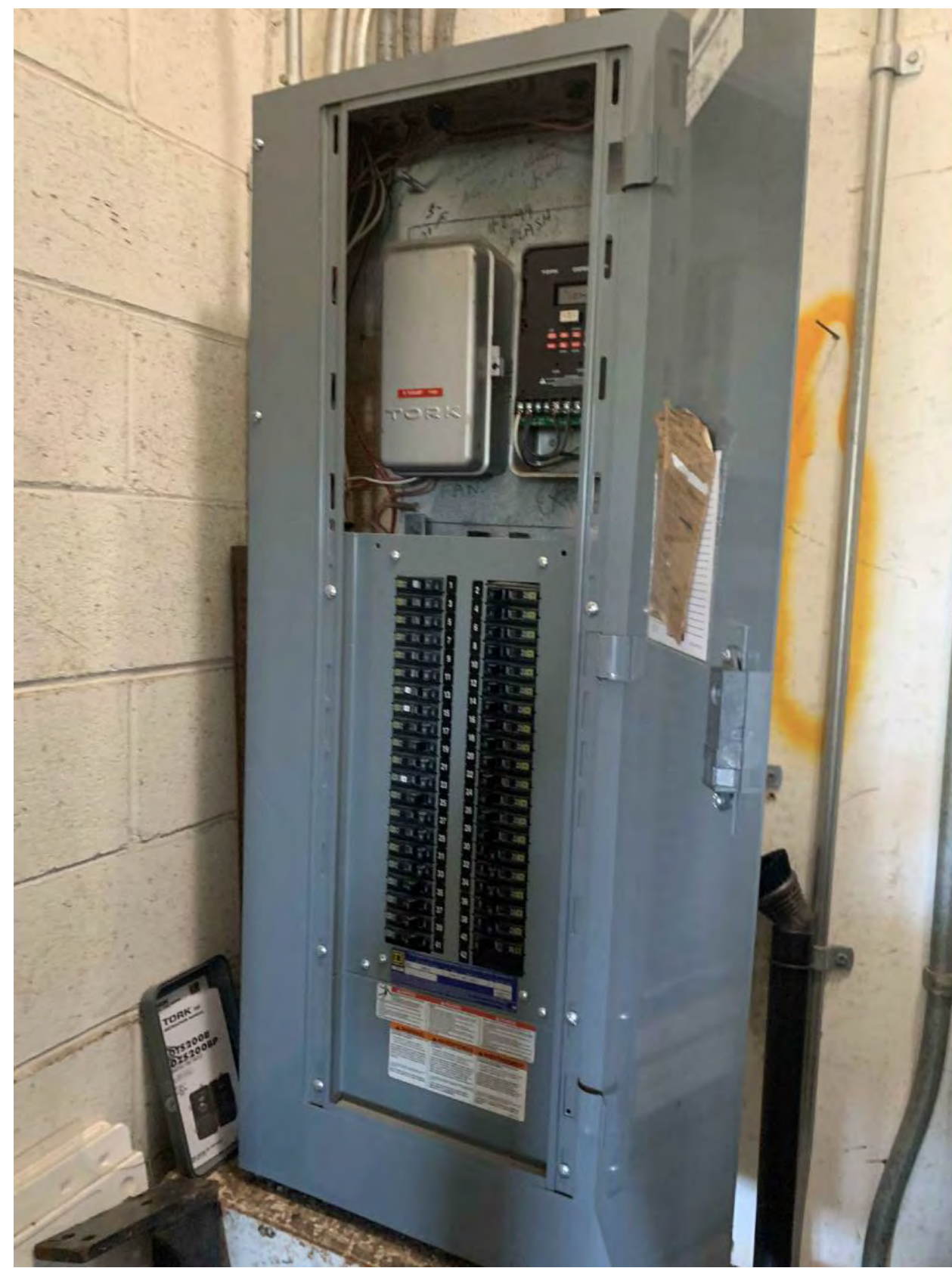
EXISTING PANEL HP1
