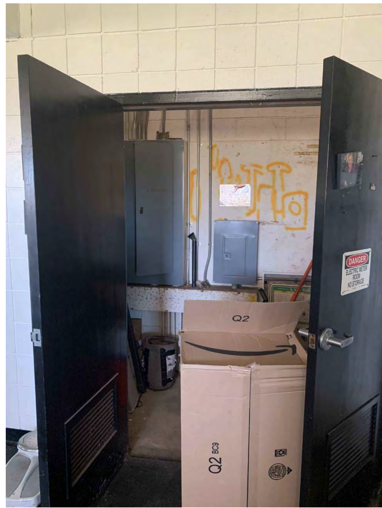
EXISTING RECREATION CENTER ELECTRICAL CLOSET
