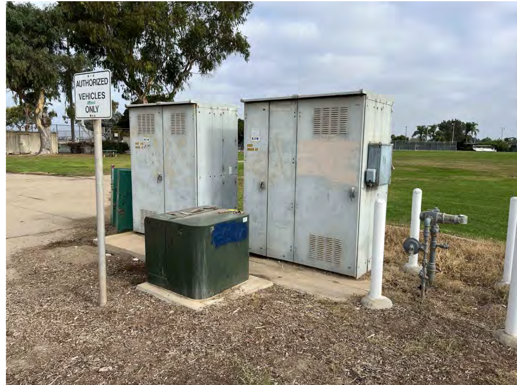
EXISTING EXTERIOR UTILITY AND DISTRIBUTION EQUIPMENT
