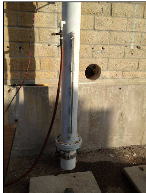
Photo 4-5: Calibration Test Equipment Configuration
