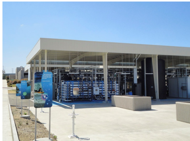
The AWP Facility produced purified water using the same processes as a potential full-scale facility.
