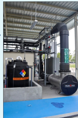
Step 3: Ultraviolet Disinfection/Advanced Oxidation
