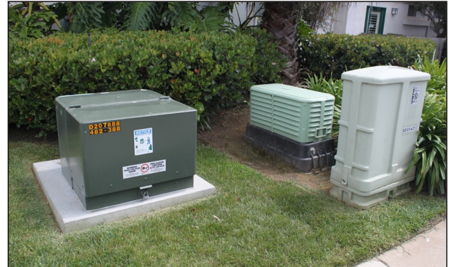
Figure 6: Transformer and cable box
