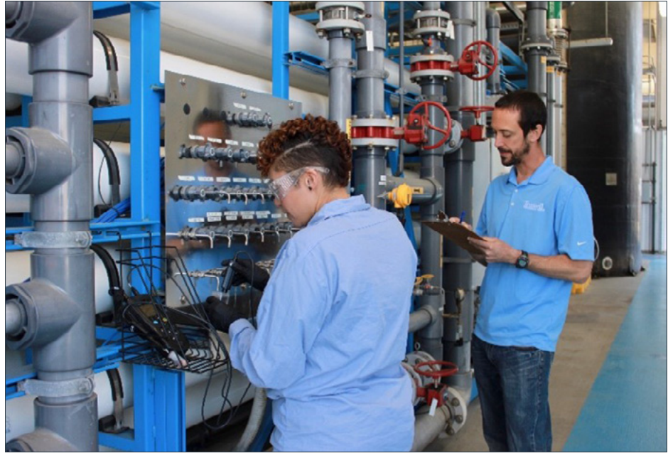
Demonstration Facility: A City team member and Pure Water consultant working together at the Demonstration Plant taking a sample of Pure Water for testing purposes
