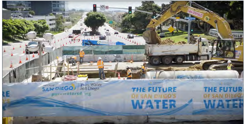
Construction in a major intersection for the Morena Northern Pipelines & Tunnels project in University City.
