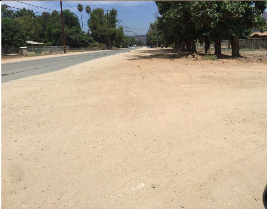
Overview photos of road ruts PWP 9 through PWP 19
