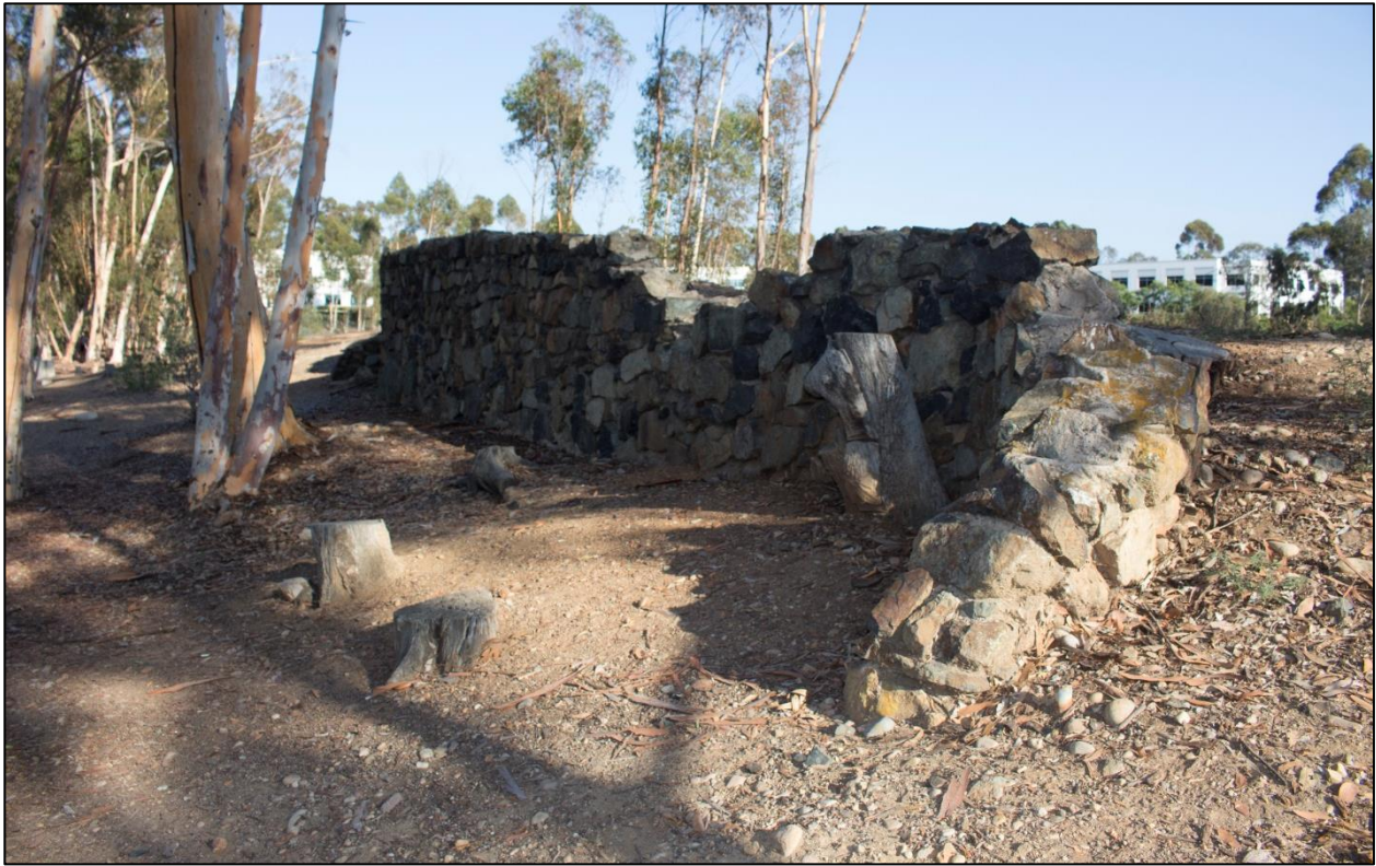
Figure 15. View of the stone wall showing missing portions, looking east-southeast (Photo credit: Dudek).
