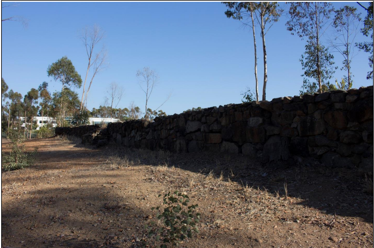
Figure 18. Length of wall; notice the large crack near center-right of the picture (Photo credit: Dudek).
