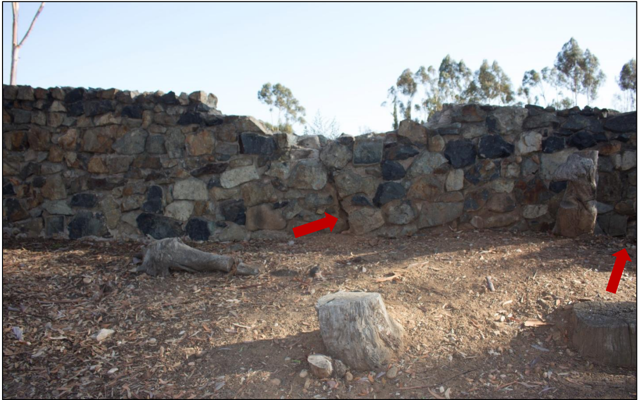
Figure 16. View of wall section showing missing portions and cracks (red arrows) (Photo credit: Dudek).
