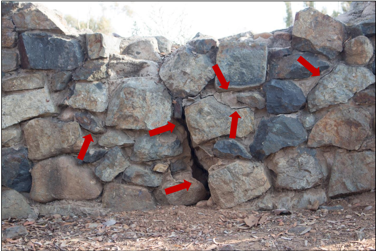
Figure 17. Detail view of above wall section showing missing portions and cracks (red arrows) (Photo credit: Dudek).
