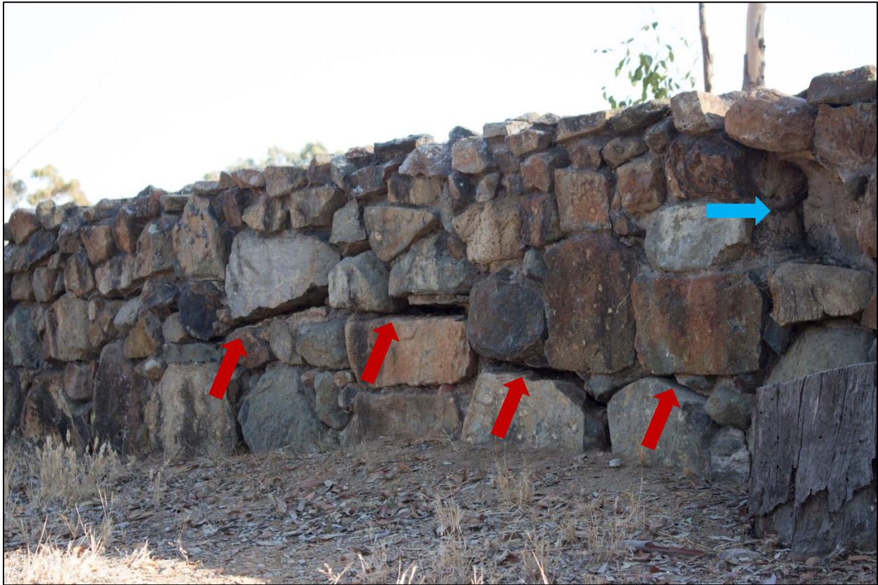
Figure 19. Detail view of above wall section showing large crack (red arrows) and a missing cobblestone (blue arrow) (Photo credit: Dudek).
