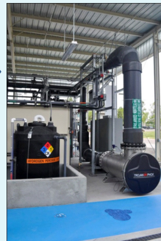
Step 3: Ultraviolet Disinfection/Advanced Oxidation
