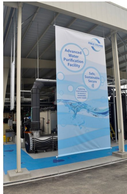
The Demonstration Facility was installed and operated to produce and test purified water.
