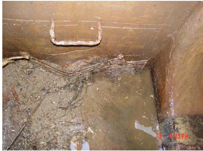
Figure I-22. Sediment and debris clogging the diversion rack at storm drain SD7-6.
