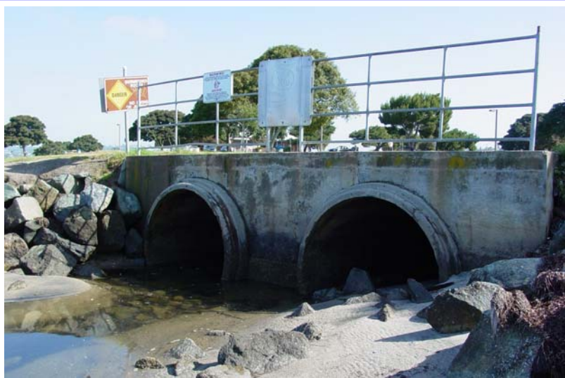
Figure I-24. Storm drains 8-1 (on left) and 8-2 (on right), located just south of the Visitor's Center building.
