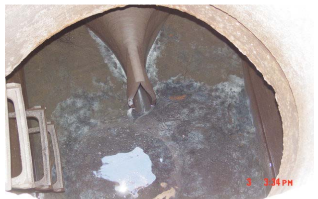
Figure I-3. Photograph of a typical tide flex valve used to prevent salt water intrusion of the diversion system. This tide flex has been bowed open and is ineffective in preventing tidal backflow.
