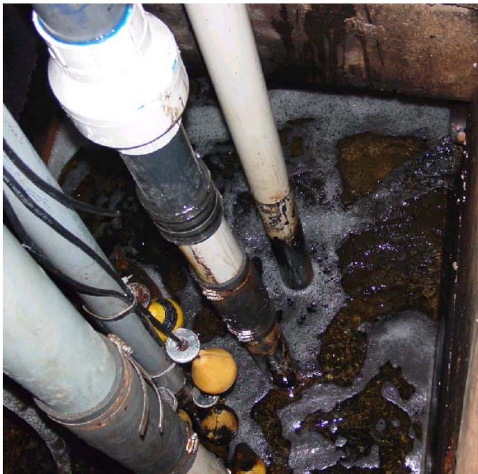
Figure I-12. De-watering sump pump located at Fanuel Park.
