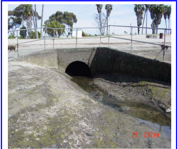
Figure I-27. Photograph of storm drain SD9-1 on the northeast side of Leisure Lagoon.
