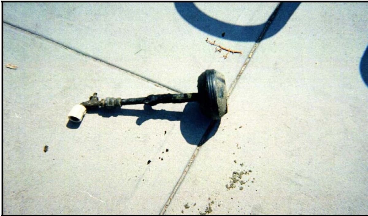
Figure I-13. Plug found after vacor truck cleaning of storm drain system.
