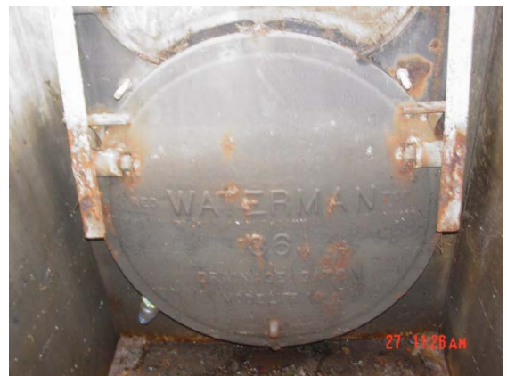
Figure I-2. Photograph of a typical flap valve used to prevent salt water intrusion of the diversion system.
