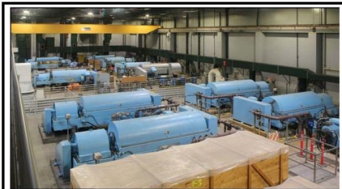
Metro Biosolids Center, Centrifuge Room Photo: Louis Rodolico 8/15/2017
