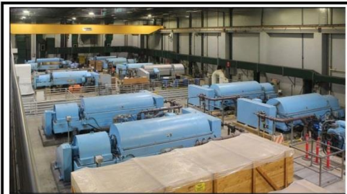
Metro Biosolids Center, Centrifuge Room Photo: Louis Rodolico 8/15/2011
