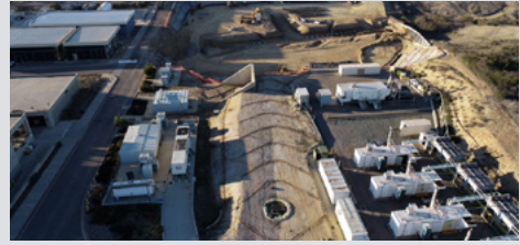
The North City Water Reclamation Plant is under construction with earth moving and site preparation. Seen here is an aerial shot looking north onto the site. (Nov. 2021)
