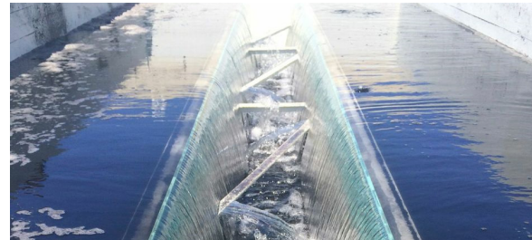
Barrier 2 Biological Activated Carbon Filters
