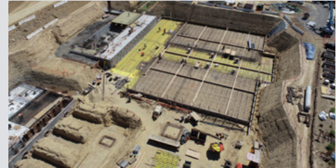
The North City Pure Water Facility project is making progress. This southwest aerial photo shows the foundation for the ozone building. (Sept. 2021)
