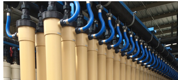
Barrier 3 Membrane Filtration
