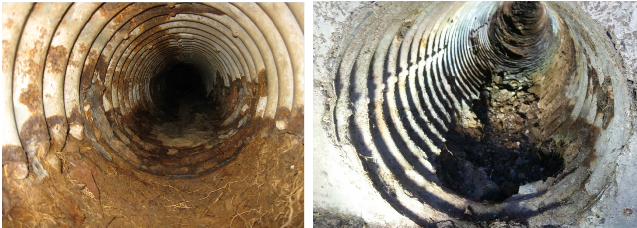
Source: Storm Water Division’s photos of deteriorated corrugated metal pipes.
