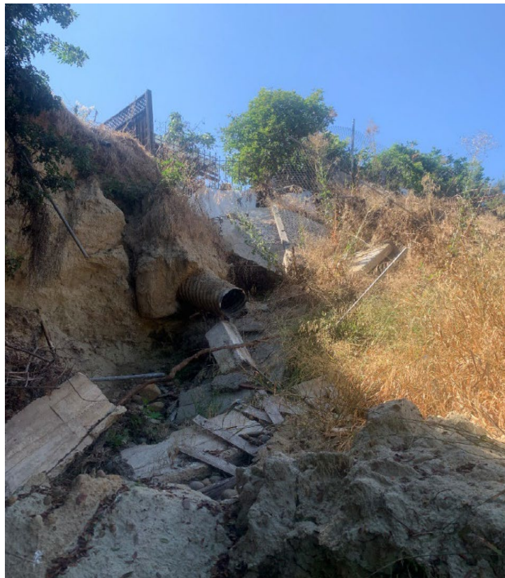
SLOPE EROSION FROM DOWNSTREAM
