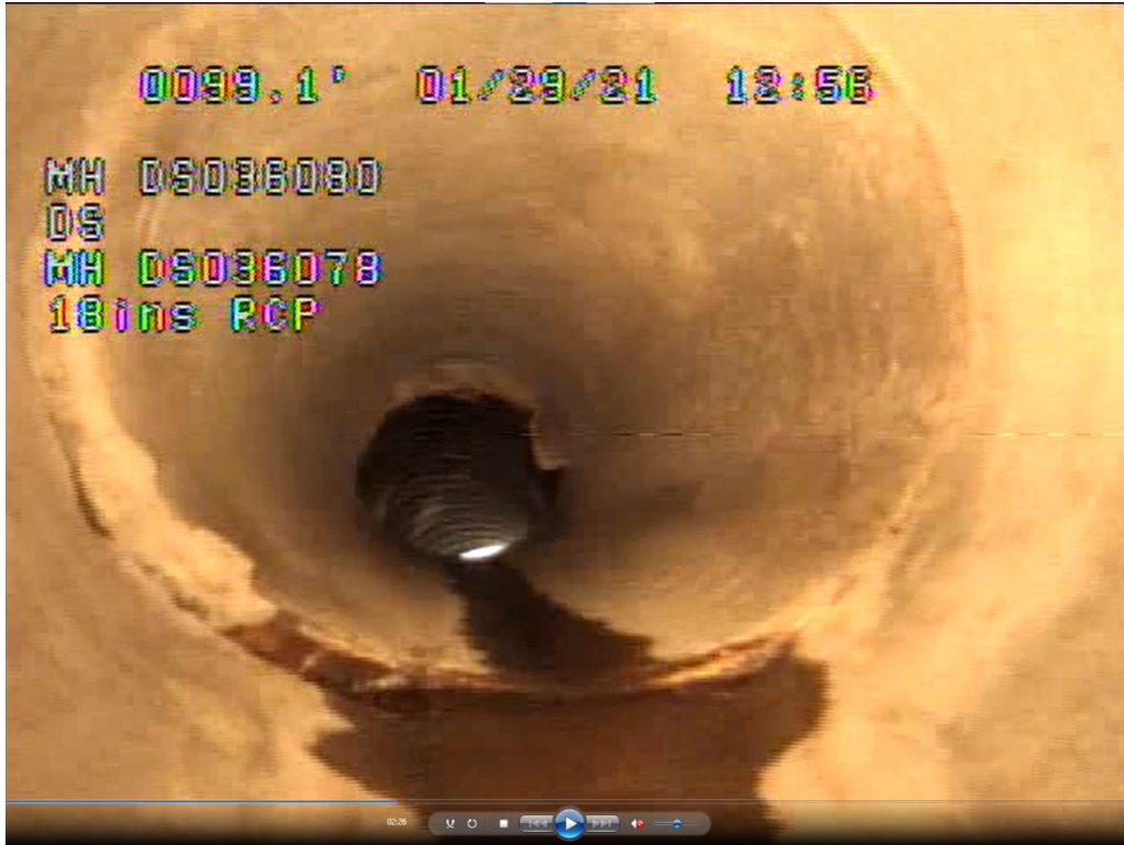
RCP OFFSET JOIN PRIOR TO FAILED CMP SEGMENT
