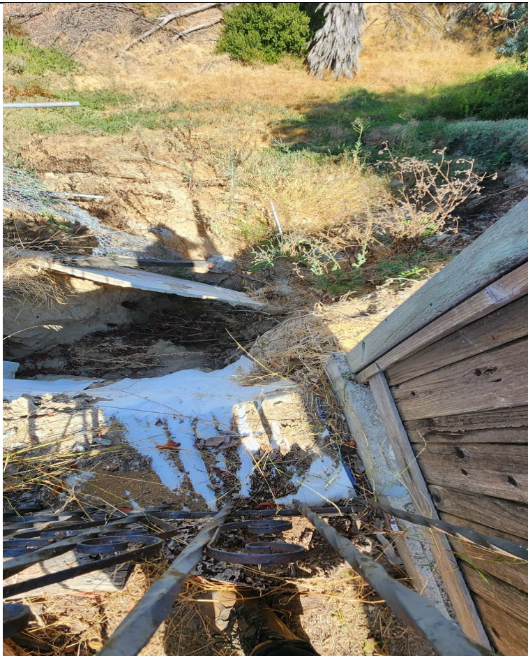
Looking down the vertical back cut of the ravine at the concrete deck, that has fallen in the ravine.
