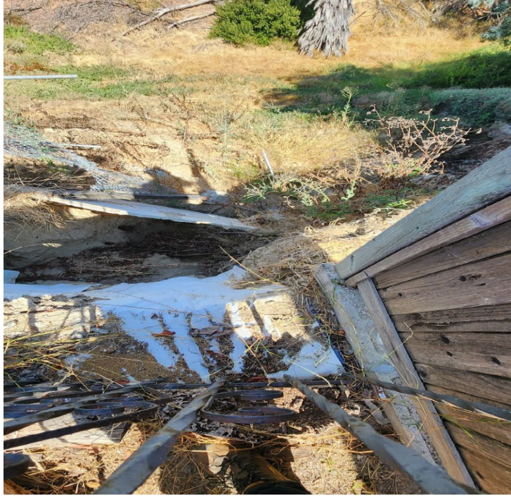
SLOPE EROSION FROM DOWNSTREAM
