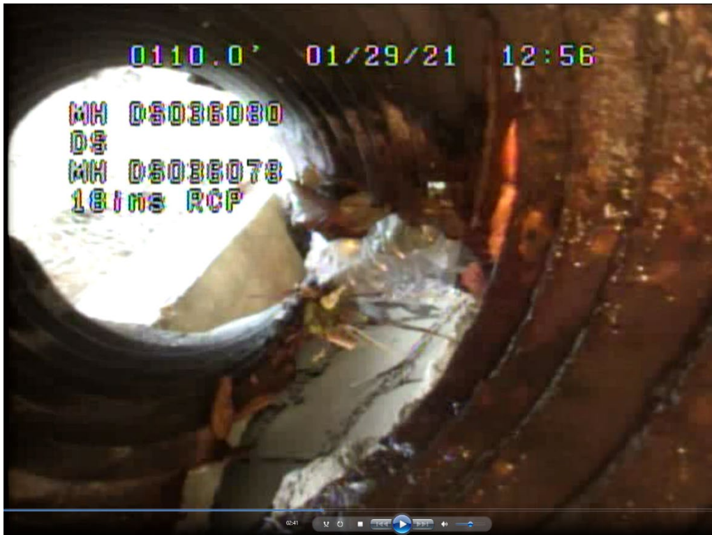
CMP AND HEADWALL FAILURE
