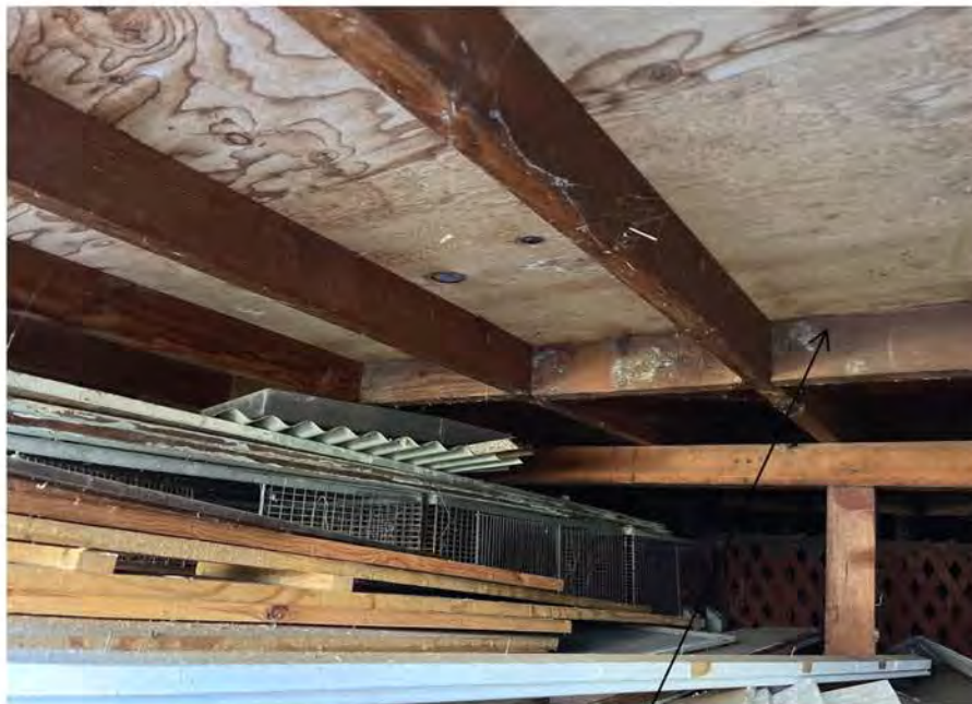
Inadequate floor structure. Replace or reinforce framing.
