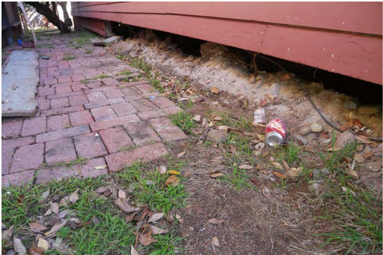
Photograph #25: North elevation, foundation crumbled away
