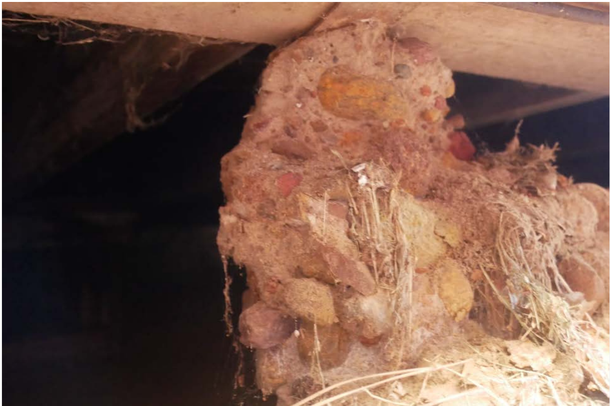
Photograph #27: North elevation, foundation crumbled away
