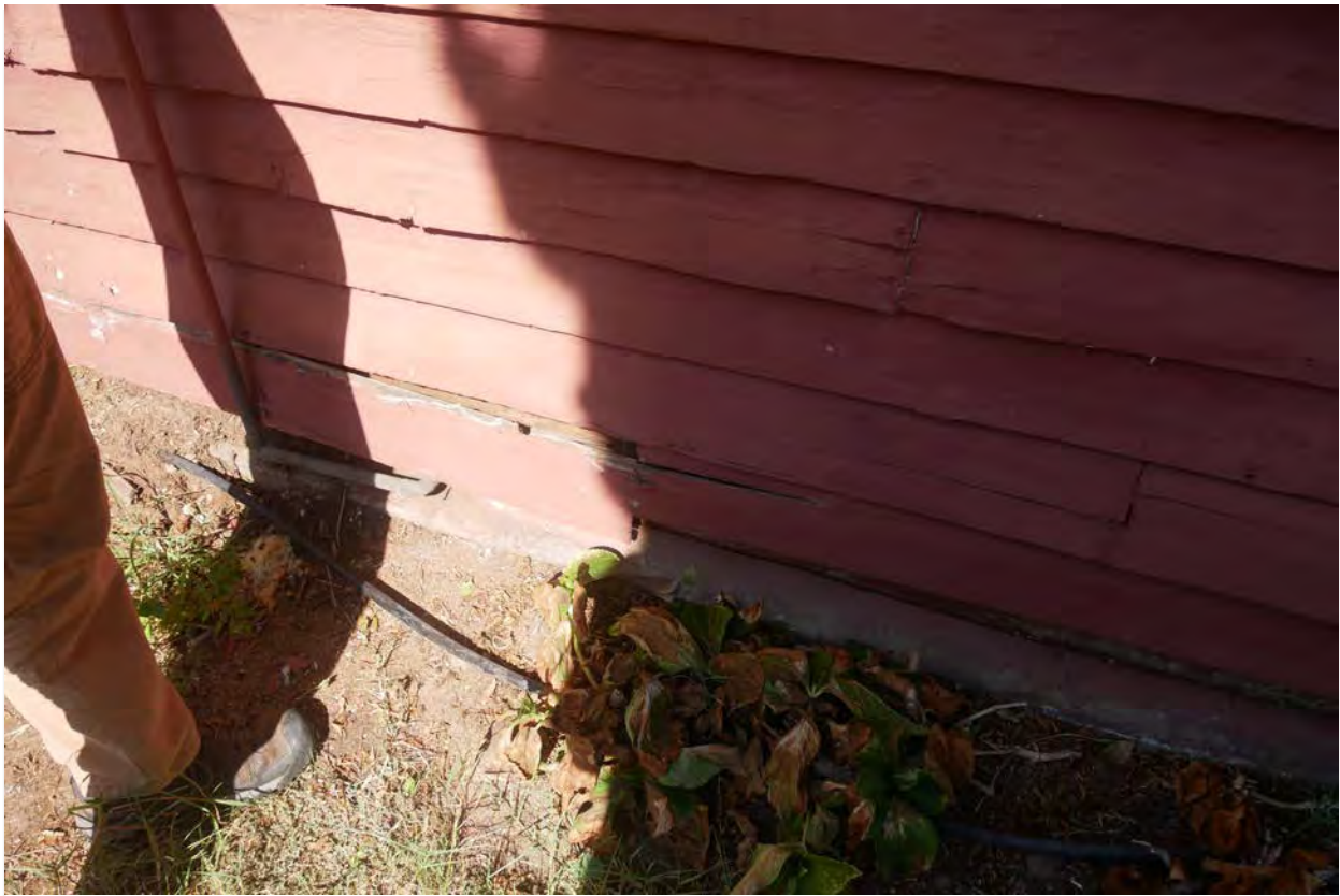
Photograph #28: South elevation, wood rot
