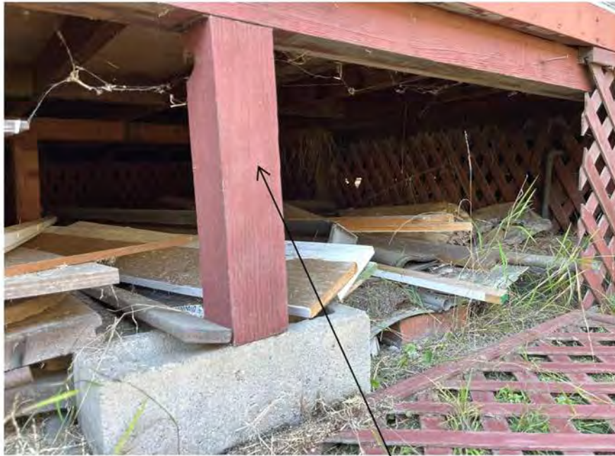
Inadequate floor structure. Replace or reinforce framing.
