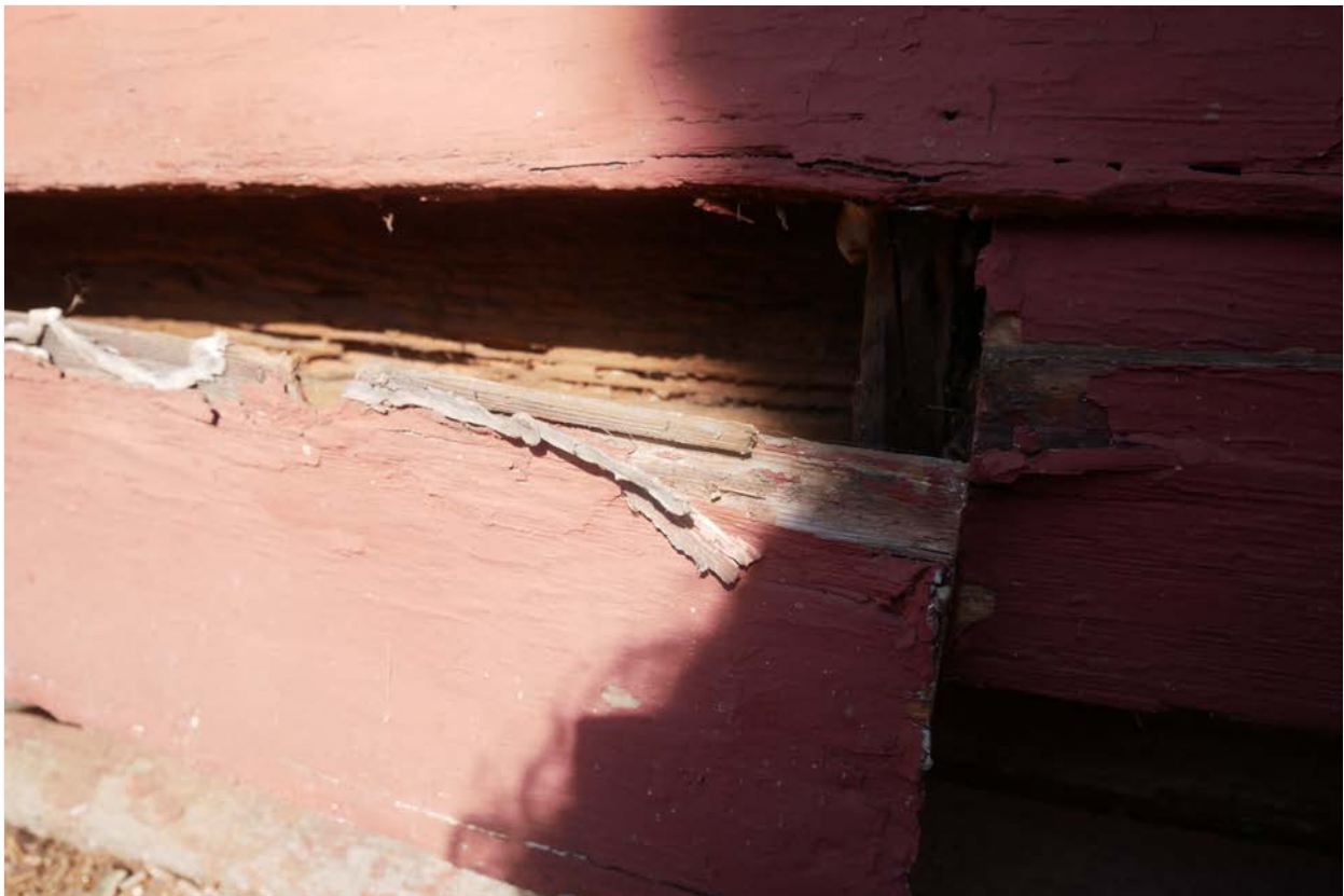
Photograph #29: South elevation, wood rot
