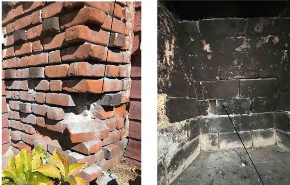
Loose & Displaced bricks. Fireboxes must be reconstructed
