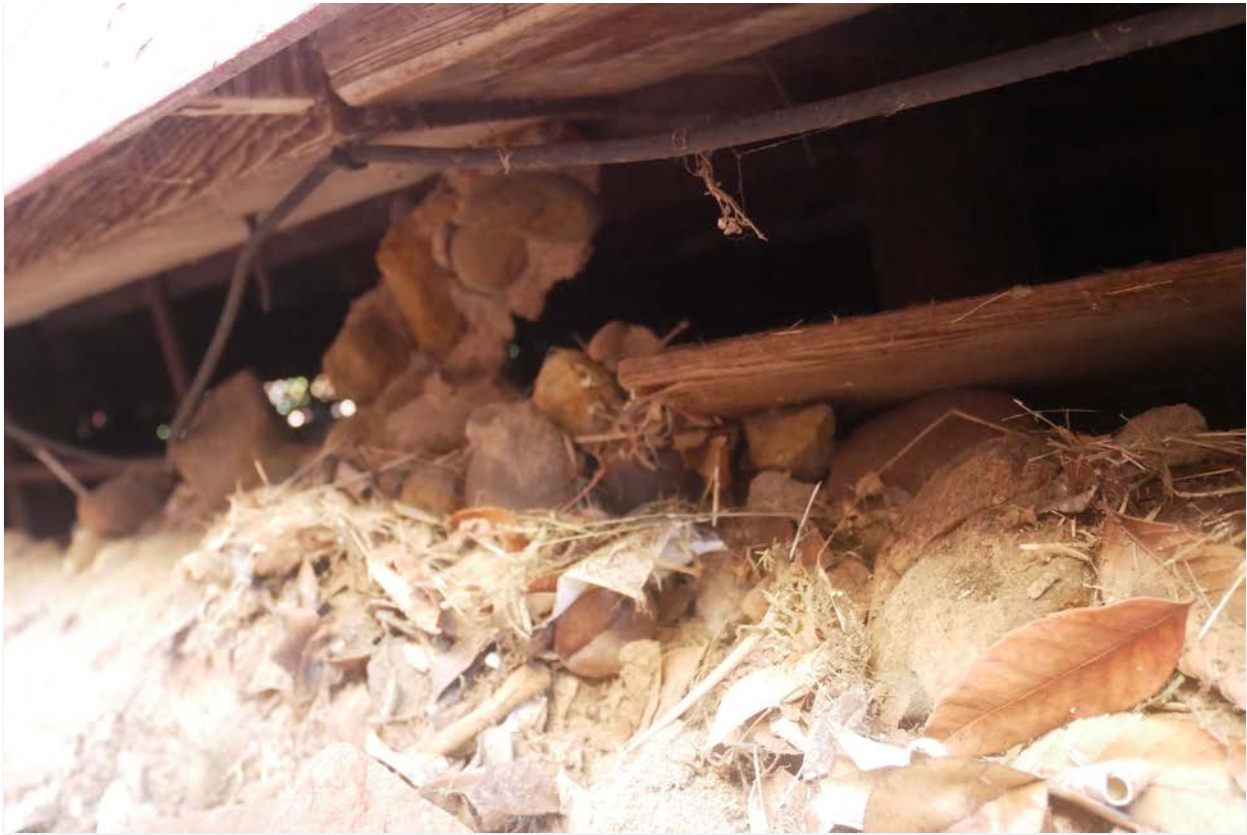
Photograph #26: North elevation, foundation crumbled away
