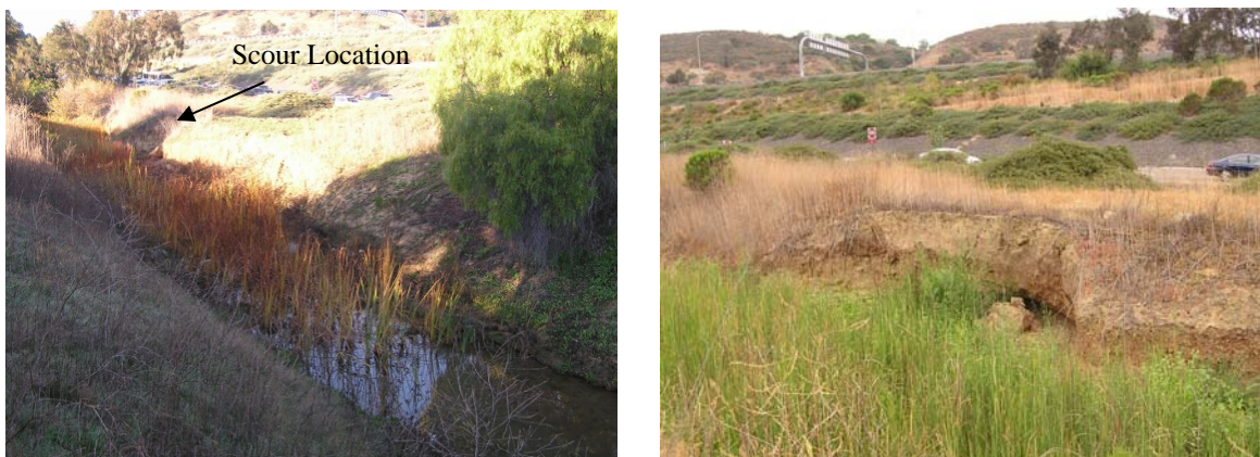
Figure 4-36. Photos of Drainage and Scour in the Lower Drainage
