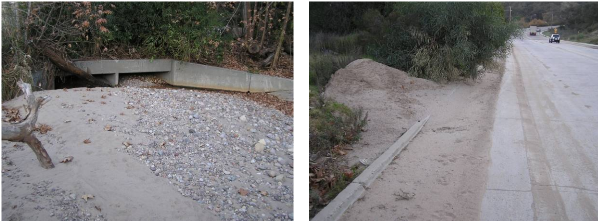
Figure 4-63. Sediment Deposition within the Culvert and along Carroll Road
