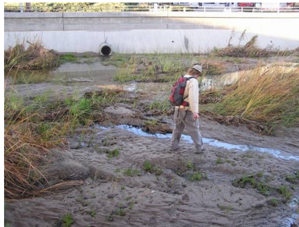
Figure ES-3. Sediment Deposition in Carroll Canyon Creek Cement Channel
