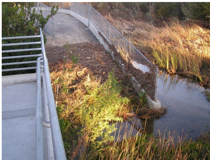
Figure 4-27. Site E, Wrack Deposition on Access Ramp
