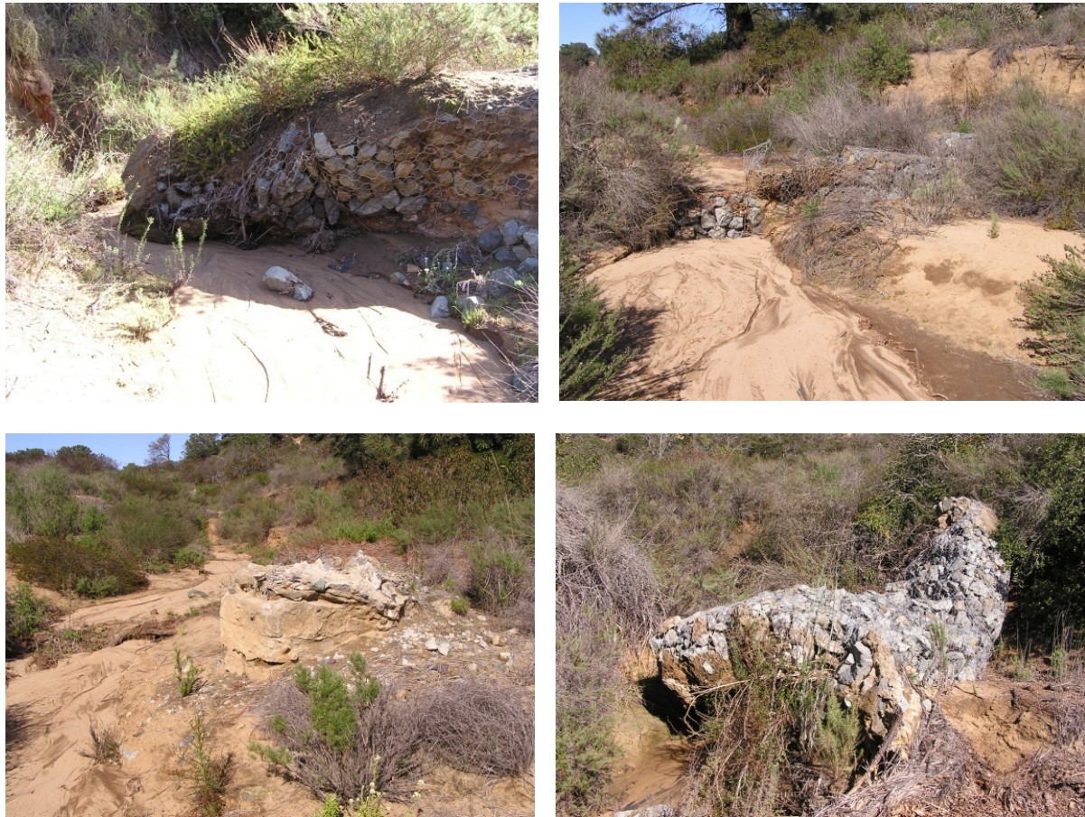
Figure 4-12. Failed Gabions within the Torrey Pines Reserve Extension
