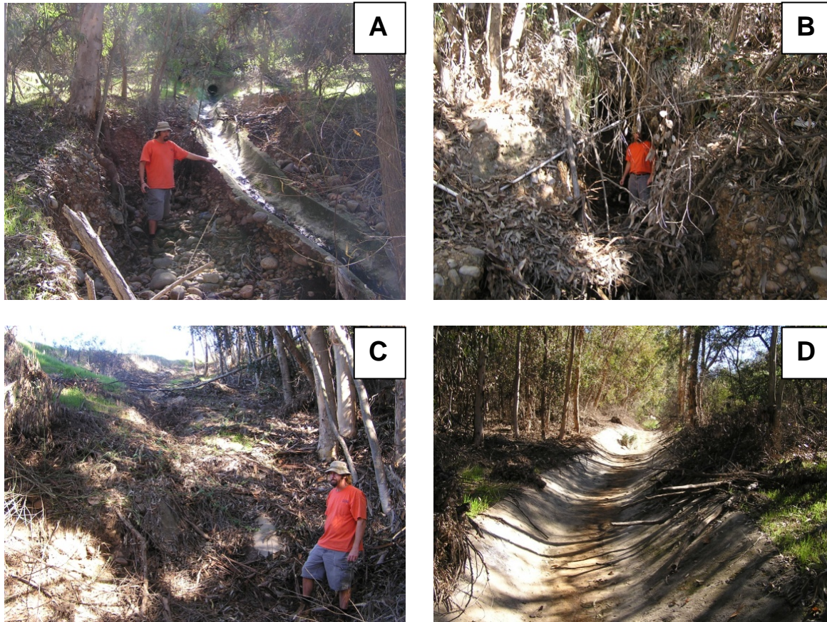
Figure 4-29. Photos of Brow Ditches in Trade Canyon
