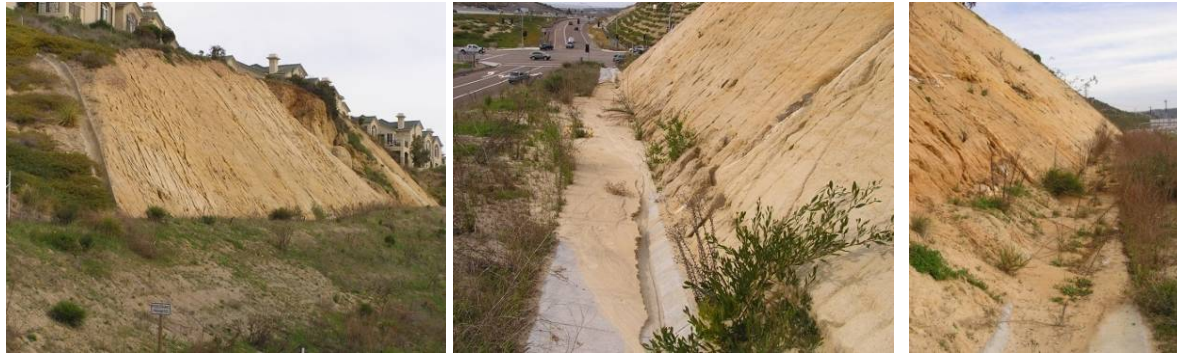
Figure 4-16. Erosion and Deposition below Torrey Villas Resort Apartments
