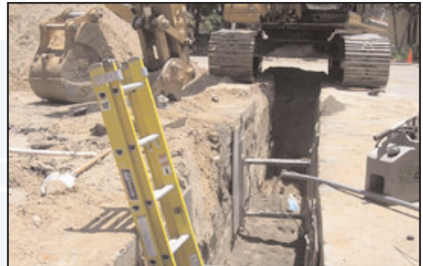
Installing 16" pipe in the northeast corner of parking lot at Seaport Village.
