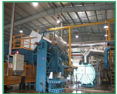
Entech Gasifier Genting, Malaysia
