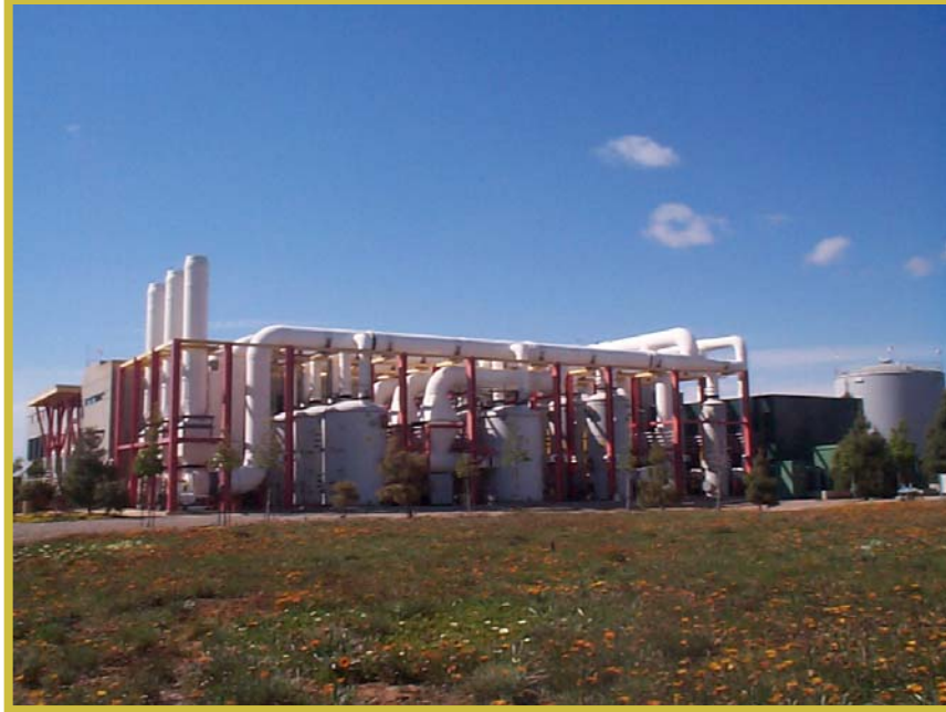
ODOR CONTROL FACILITY
