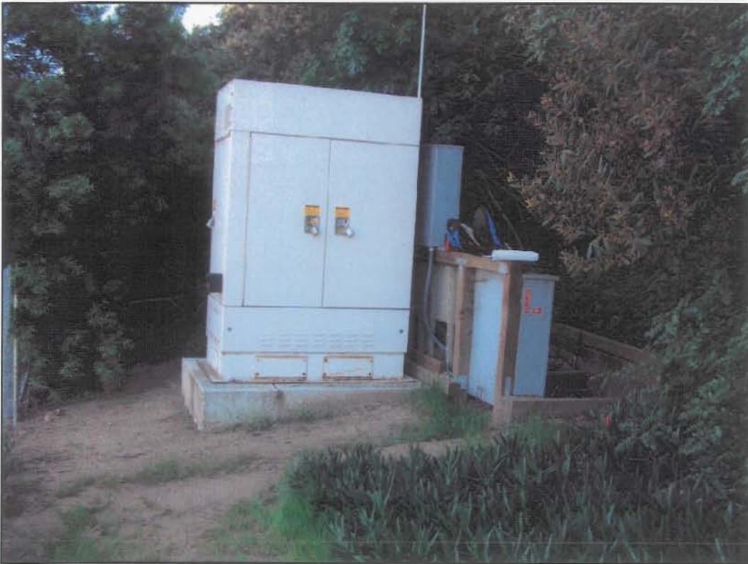
Existing equipment cabinet
