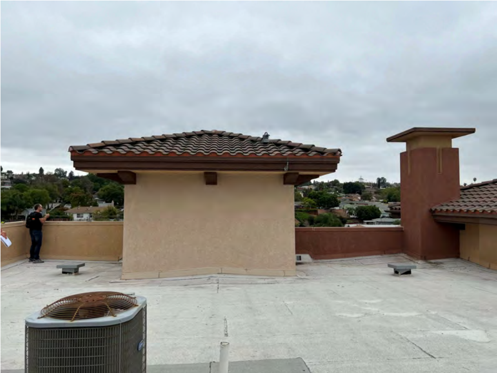
Rooftop Equipment Location
