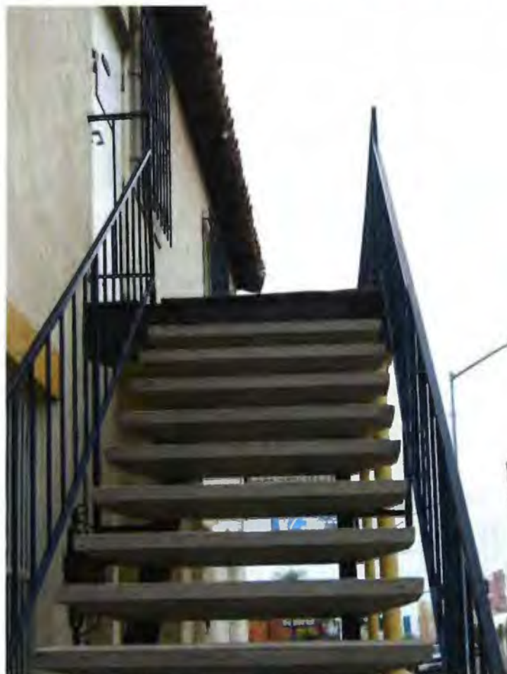
4061 Fairmont Avenue March 2017 Photograph #6 View of staircase leading to second story entrance on the West façade
