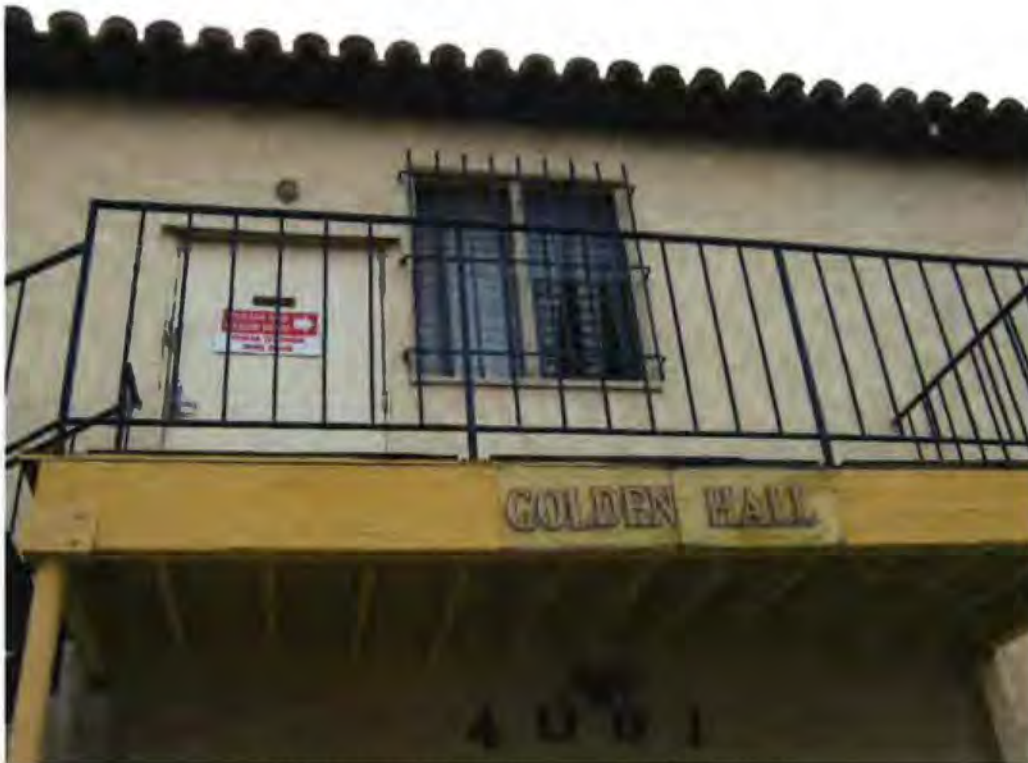
4061 Fairmont Avenue March 2017 Photograph #5 View of second story balcony on the West façade
