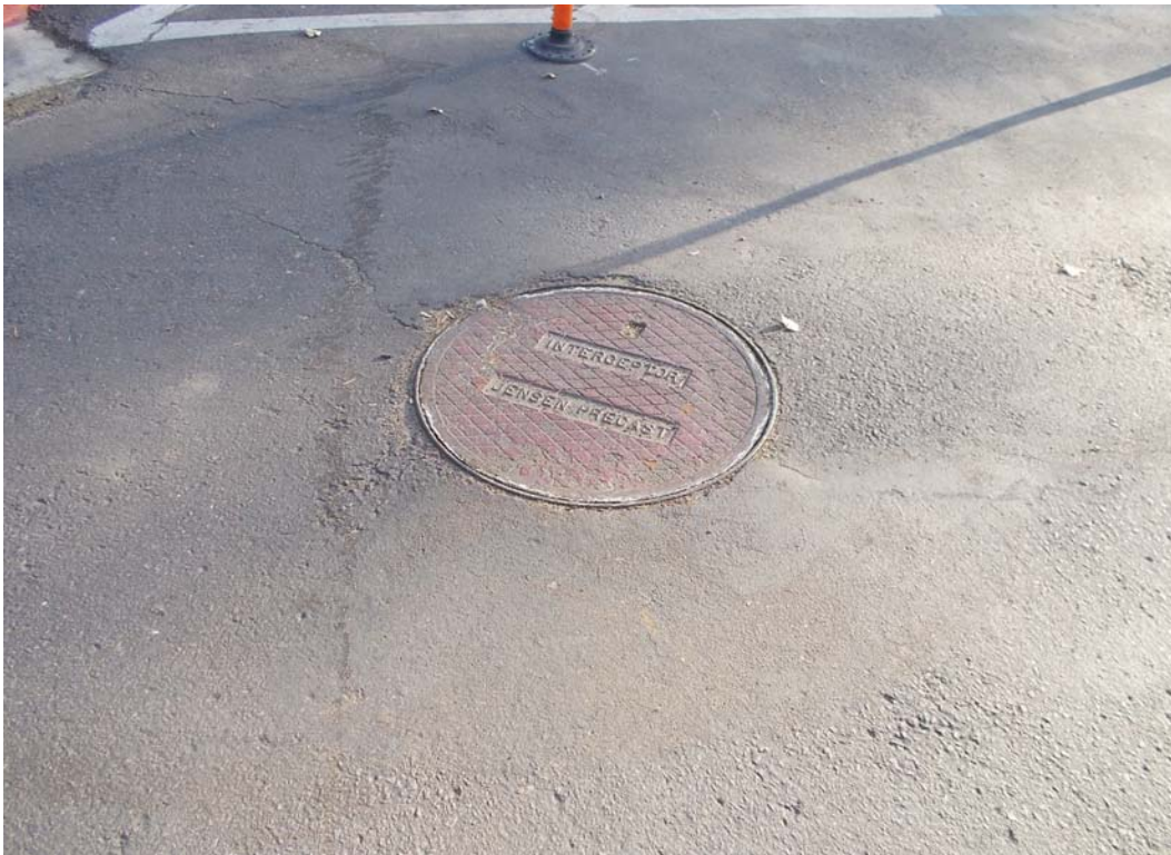
2) View of the below-ground grease interceptor located within the parking area.
