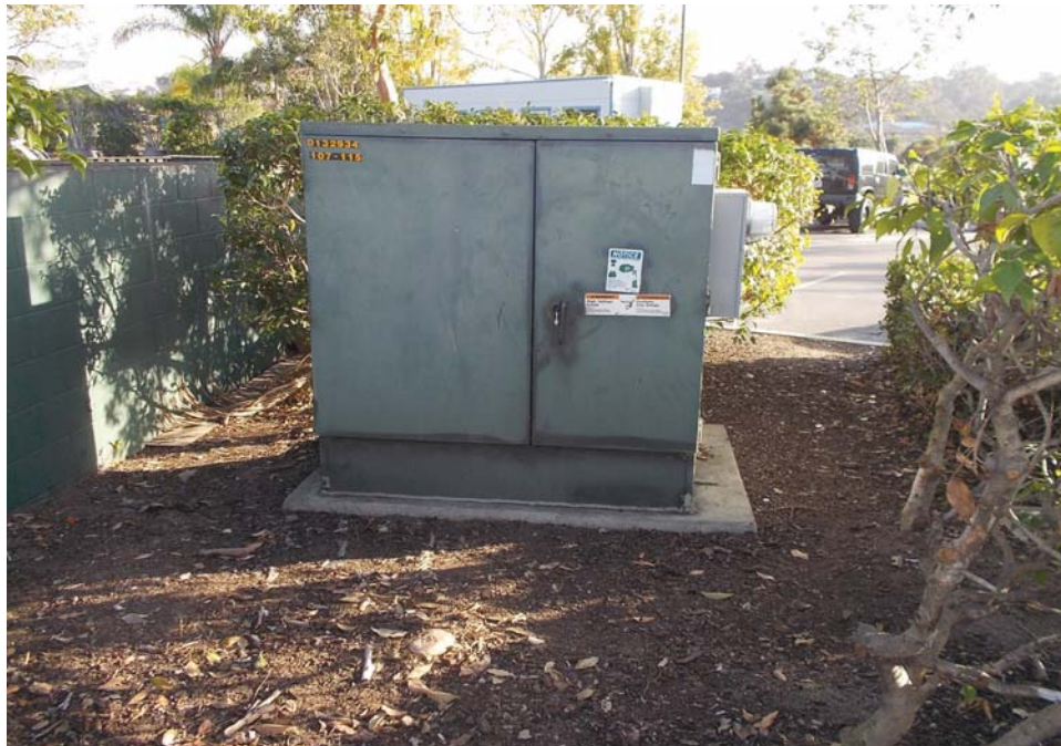
2) View of a transformer observed on Site.
