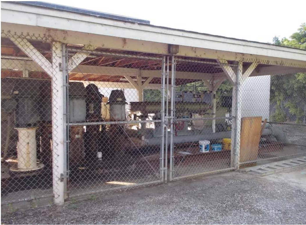
1) View of the water pump station observed at the southeastern portion of the Site.
