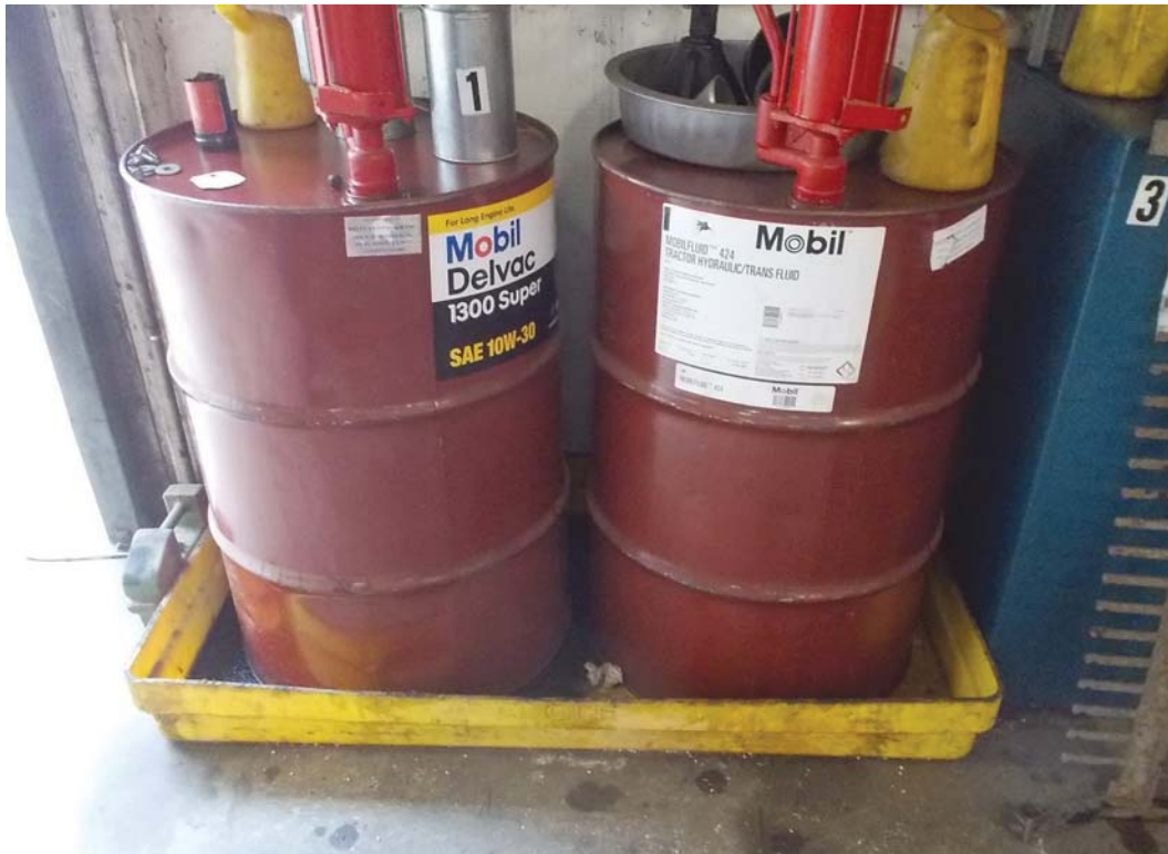
1) View of the hydraulic and transmission oil stored within the maintenance area.
