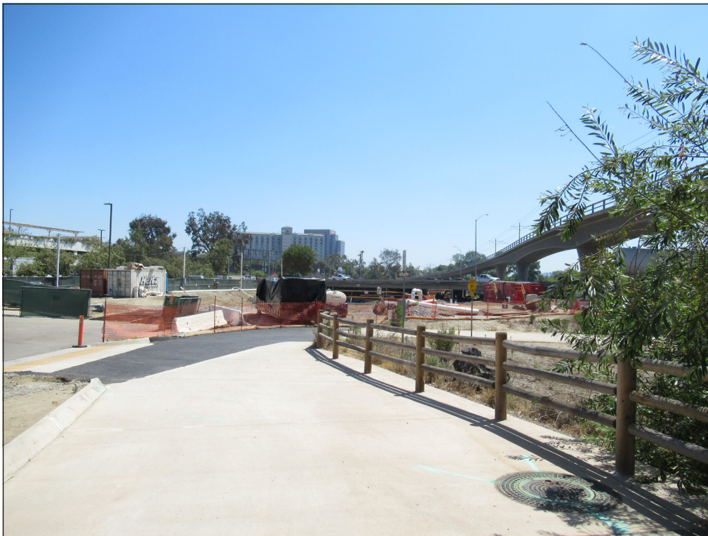
Photo 7. Laydown yard to the west of SR 163 in Fashion Valley Mall. Looking northeast.
