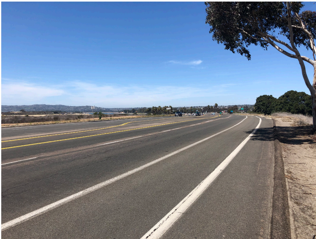
Photo 4. Northern portion of Sea World Drive, north of Friars Road, where the 12-inch water main will be constructed within the existing road right-of-way. Looking northwest.
