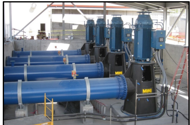
Low-Lift Pump Station
