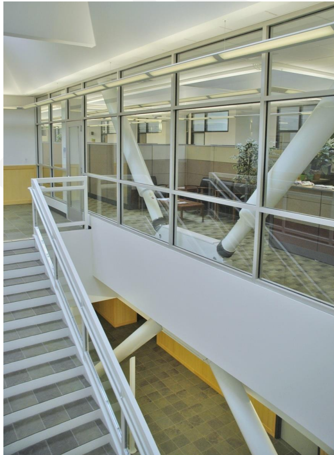
Figure 16. Viscous damper installed in a California building
