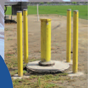
Groundwater Monitoring Well
