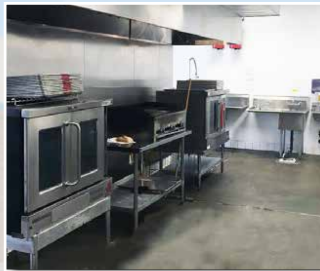
Commercial kitchen with equipment Photo courtesy Hollister Kitchens
