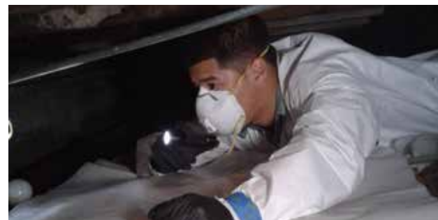
Touchet inspects pipes beneath a Smart Home Photo courtesy Urban Corps of San Diego County
