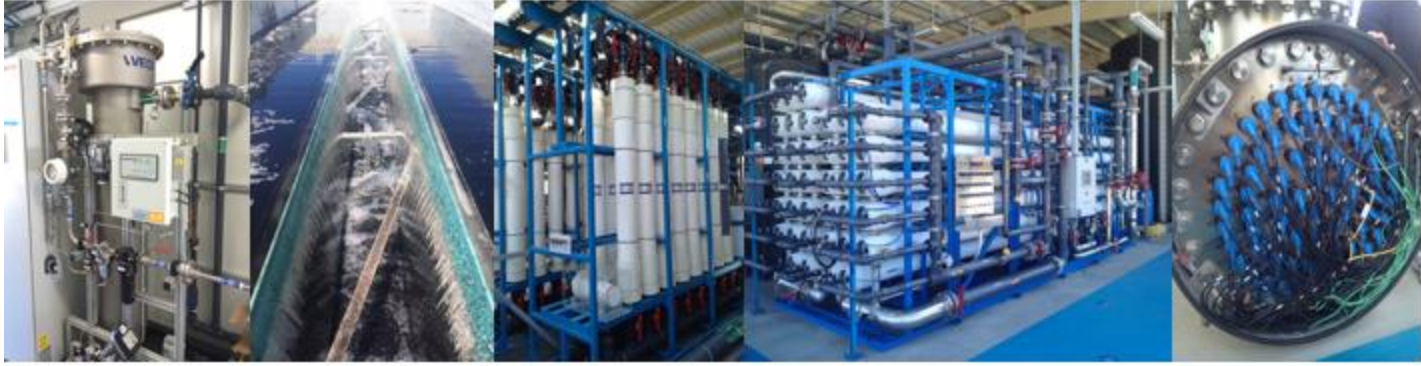
Figure 2. Pictures of the different treatment steps at 1MGD Pure Water Demonstration Facility.
