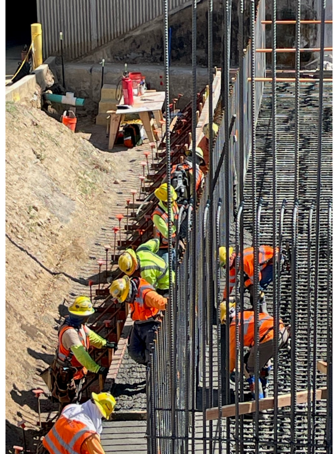
North City Pure Water Reclamation Plant Expansion and Influent Pump Station
