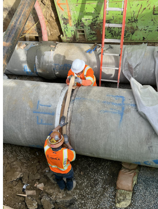
Workers constructing the pipeline from Appleton Street to State Route 52. This section is now complete and workers are moving northbound on Genesee between State Route 52 and Governor Drive through November 2023.
