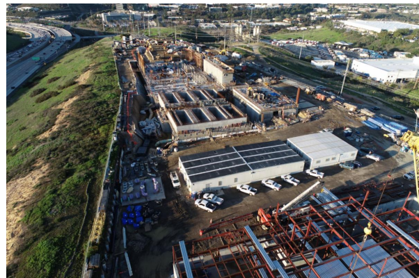
Construction at the North City Pure Water Facility & Pump Station is well underway (looking northward onto the project site; I-805 is located to the left).
