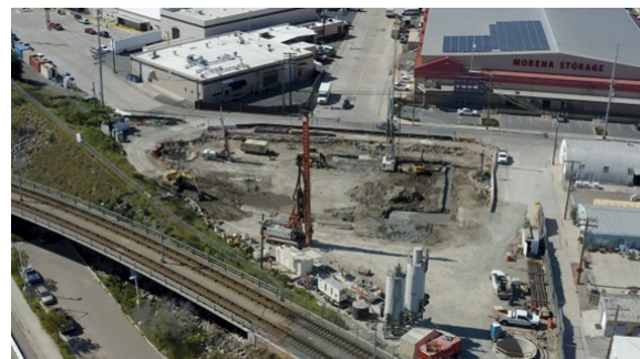
The Morena Pump Station project, at the intersection of Sherman and Custer Street.
