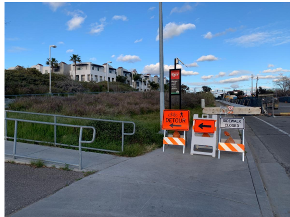
The pedestrian and bike lane detour is in place for the Morena Pump Station project.
