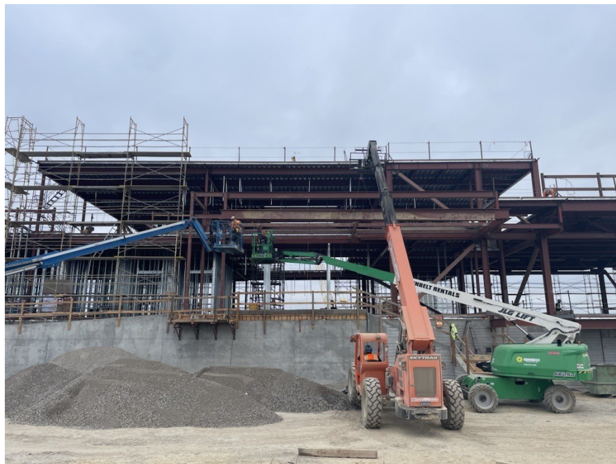
Installation of the final steel beam at the North City Pure Water Facility and Pump Station.
