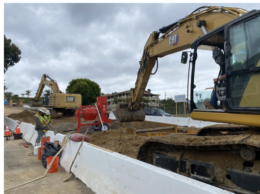
Pipeline construction is ongoing on Clairemont Drive for the Morena Conveyance South & Middle and Bikes lanes project.
