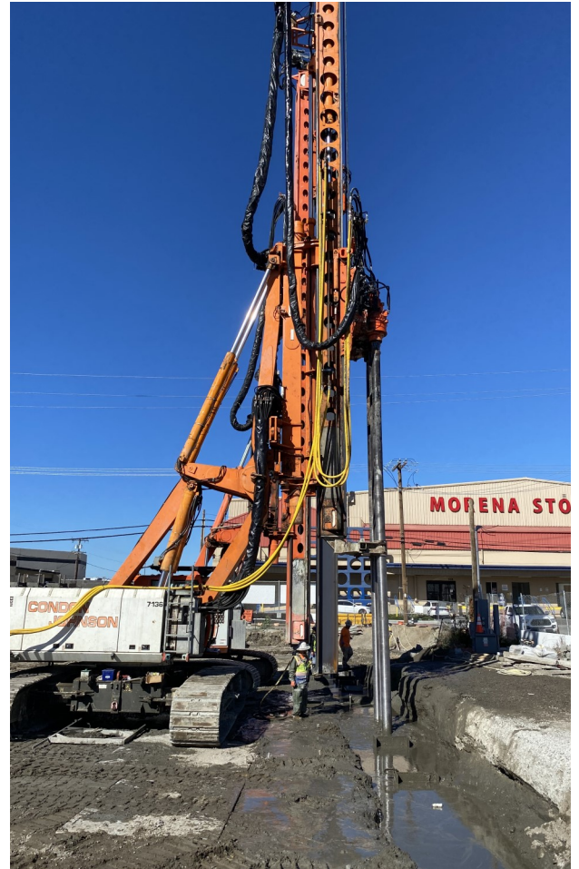
Morena Pump Station
