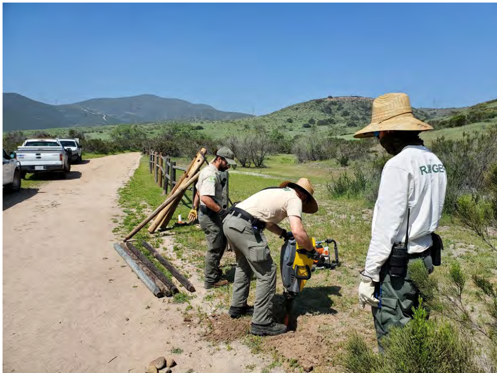
Photo 43. Fence relocated outside vernal pool.
