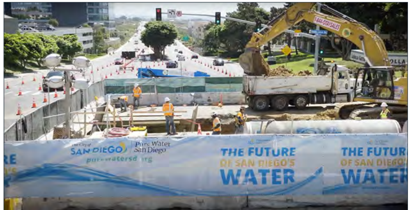
Construction in a major intersection for the Morena Northern Pipelines & Tunnels project in University City.
