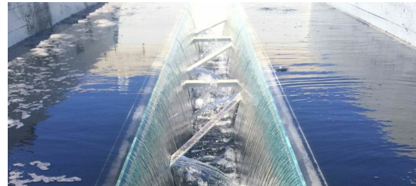
Barrier 2 Biological Activated Carbon Filters
