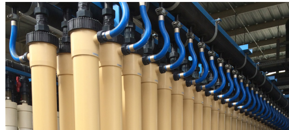
Barrier 3 Membrane Filtration
