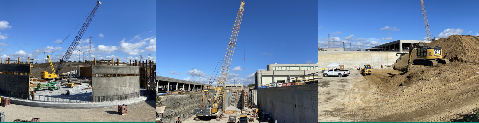
North City Water Reclamation Plant Expansion and Influent Pump Station
