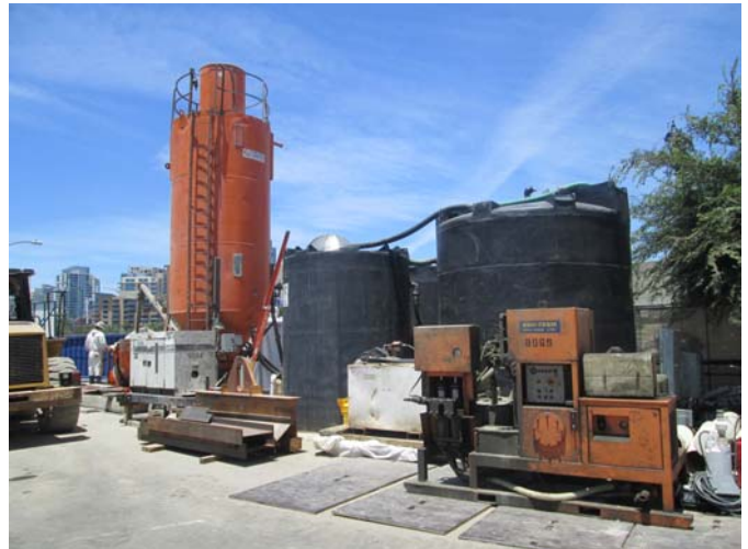
10. Dewatering treatment tanks.
