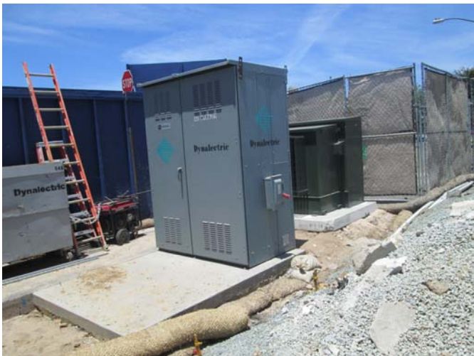
11. Utility systems on-site.
