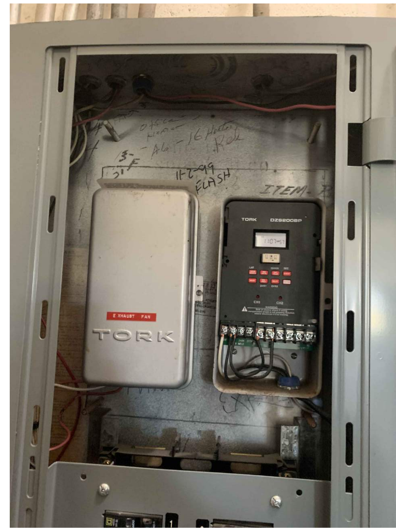
EXISTING PANEL HP1 LIGHTING CONTROLS
