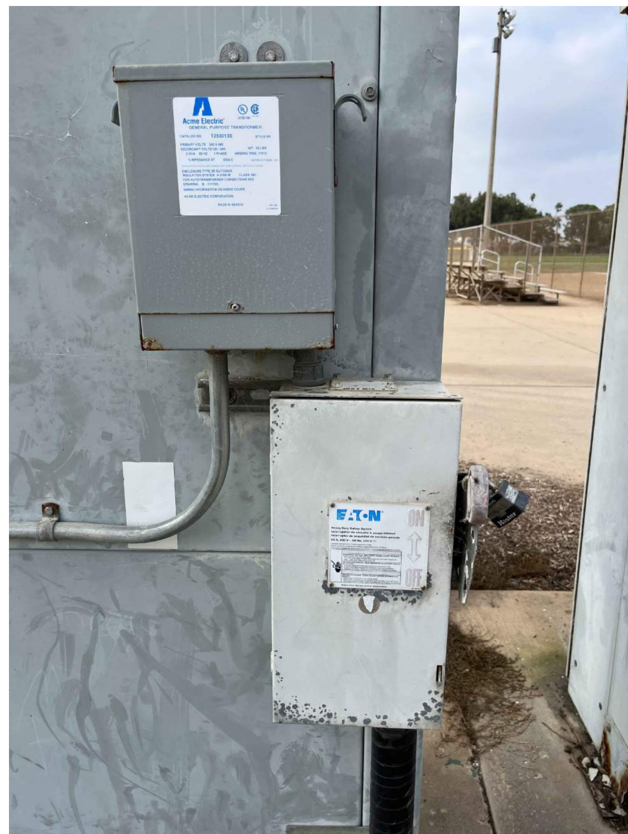
BACK OF EAST GEAR
