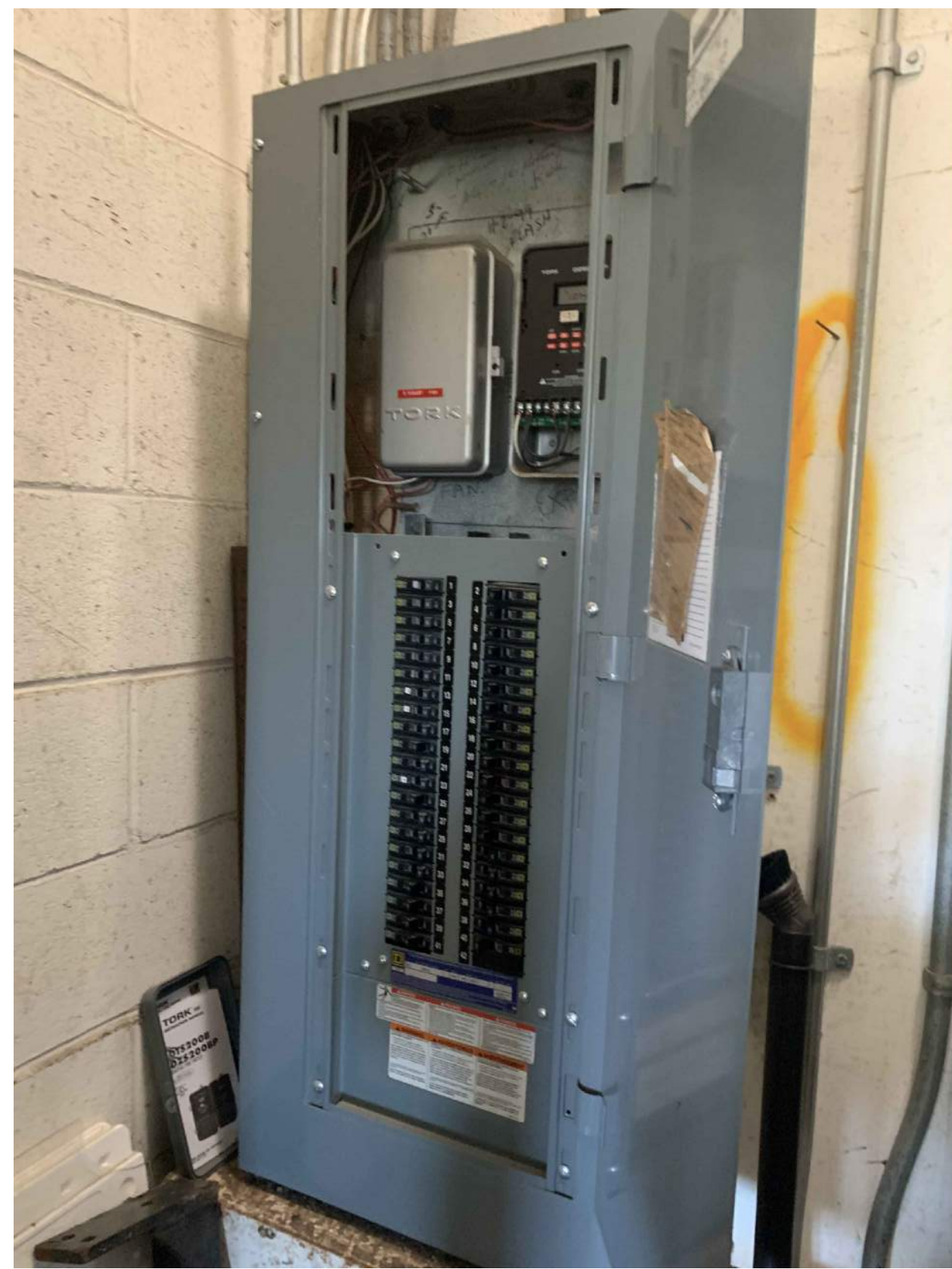
EXISTING PANEL HP1
