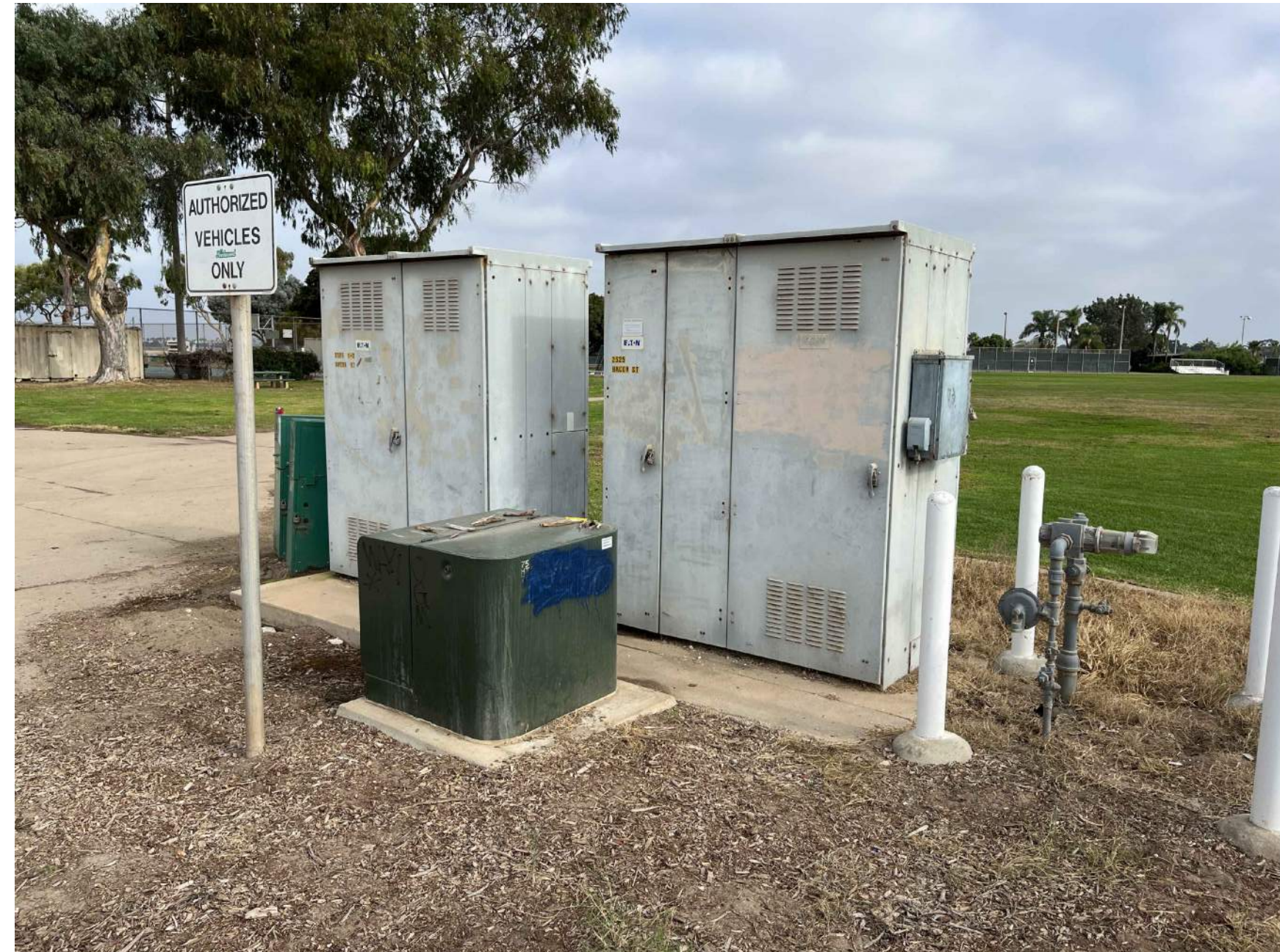
EXISTING EXTERIOR UTILITY AND DISTRIBUTION EQUIPMENT
