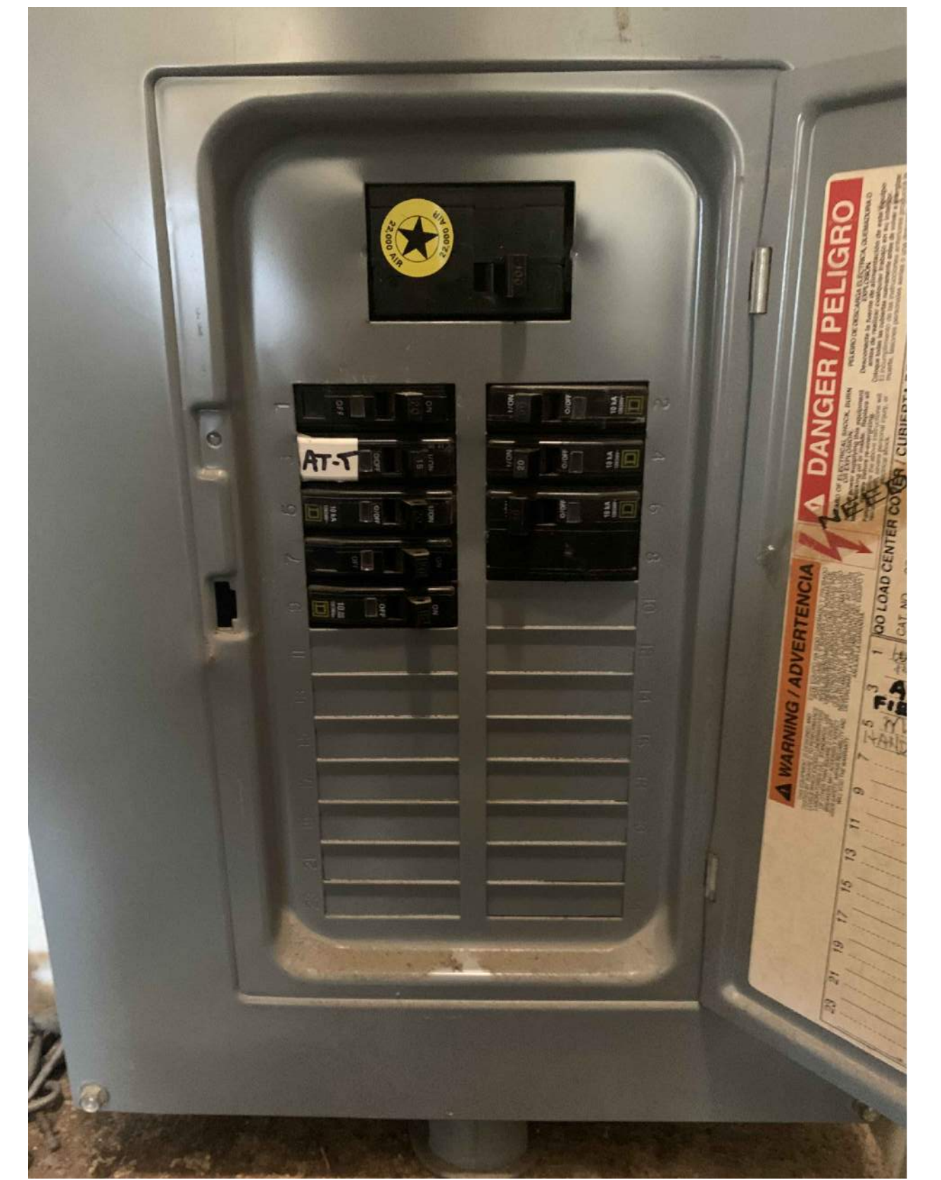
EXISTING PANEL HP2
