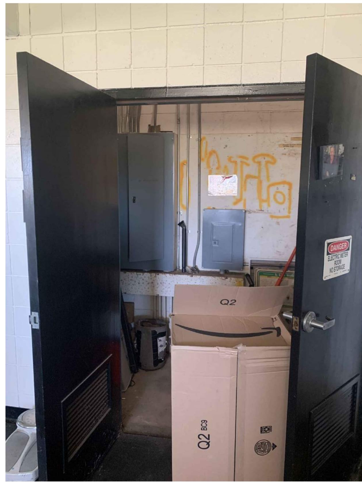
EXISTING RECREATION CENTER ELECTRICAL CLOSET
