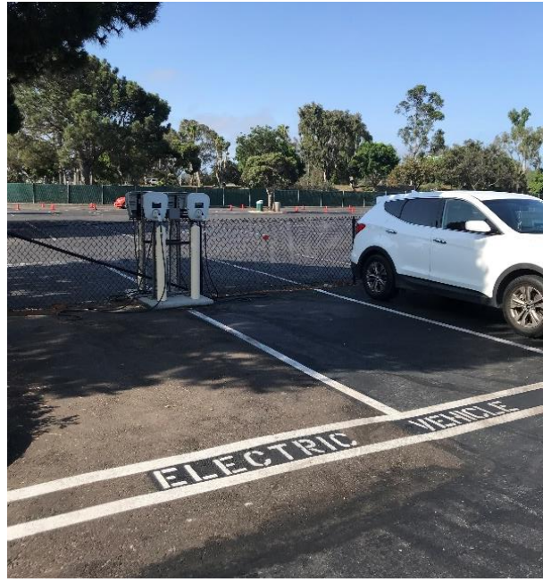
Electric vehicles charging stations
